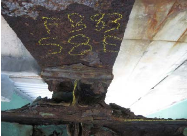
Figure 2.1: Section Loss and Web Crippling at Deck Joint
