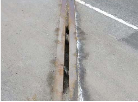
Figure 2.13: Damaged Pourable Seal
