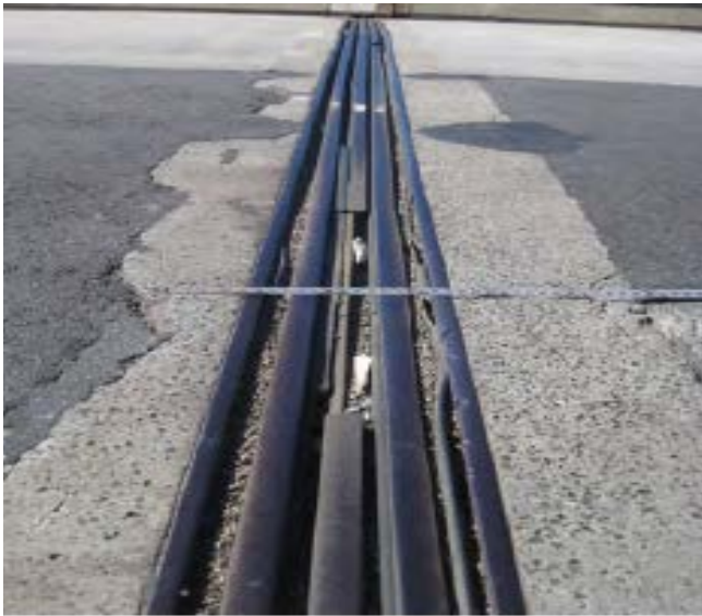
Figure 2.15: Damaged Modular Joint
