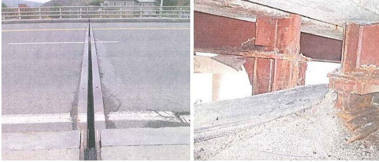
Figure 2.7: Damaged Compression Seal
