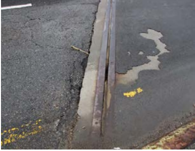
Figure 2.9: Damaged Strip Seal
