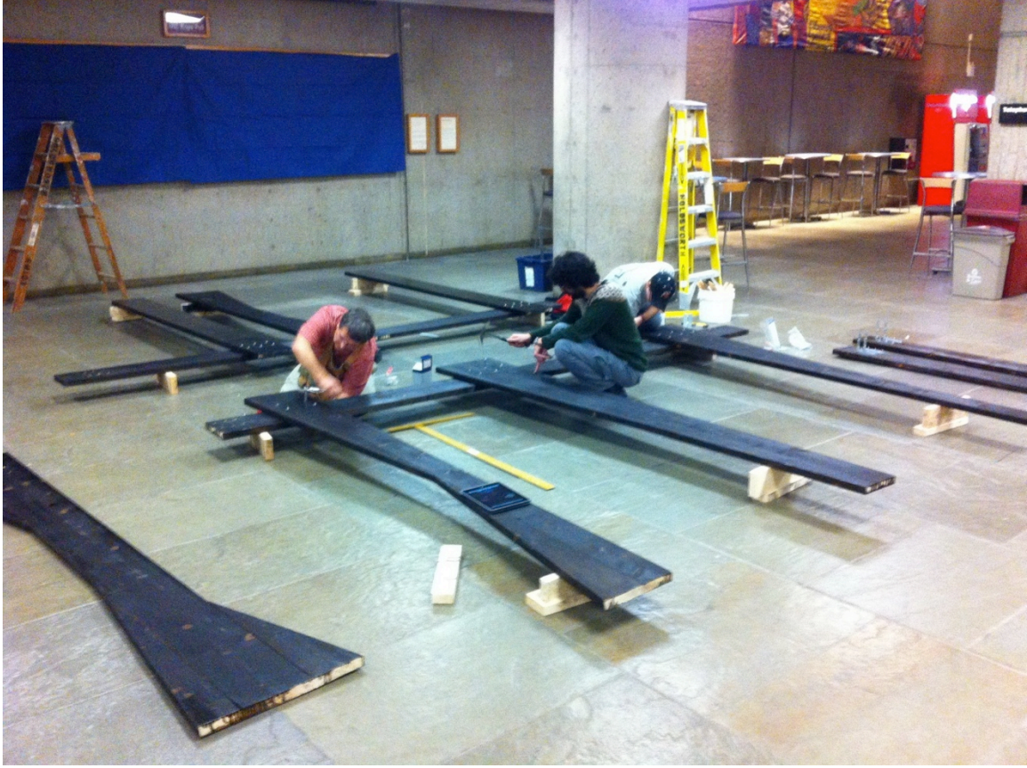
Figure 4.4: Columns on each side of the structure were put into position and bolted down to a beam before final assembly of beams together (Image credit by the Author)
