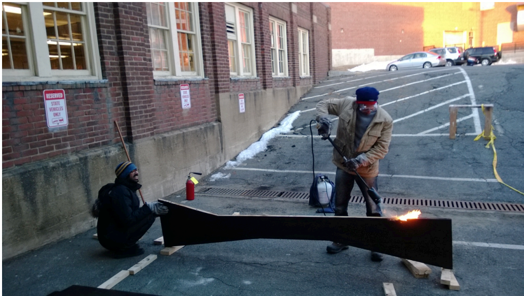
Figure 4.2: Torching structural elements using Inferno Propane Torch Kit (Image credit by the Author)
