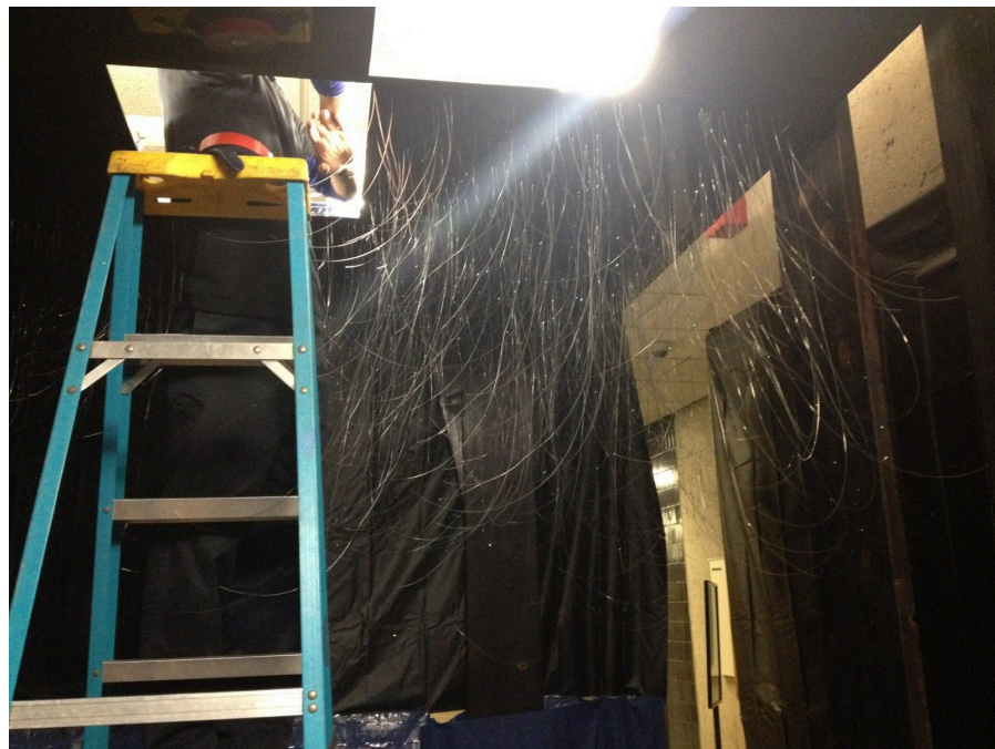
Figure 4.9: Placement of drop ceiling panels with suspended fiber optics (Image credit by the Author)
