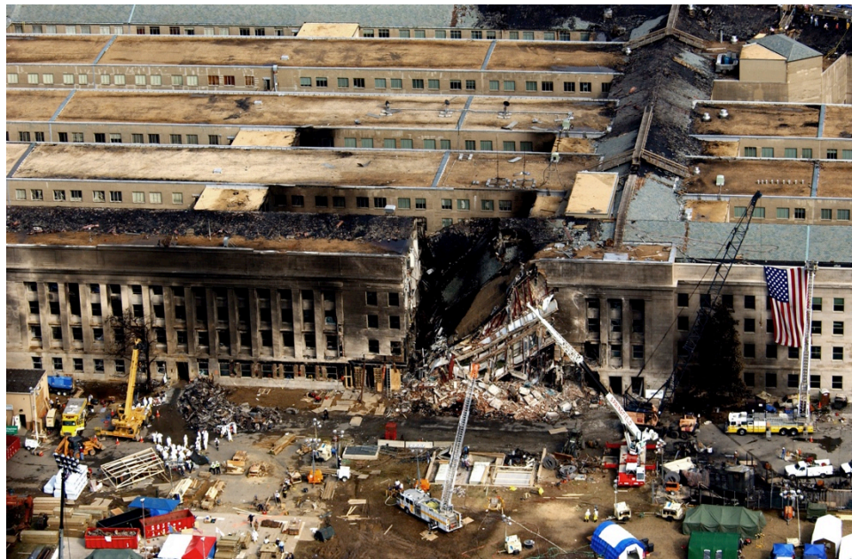
Figure 1.9: The southwestern part of the Pentagon Building targeted by the American Airlines Flight 77 (Rudisill, 2001)
