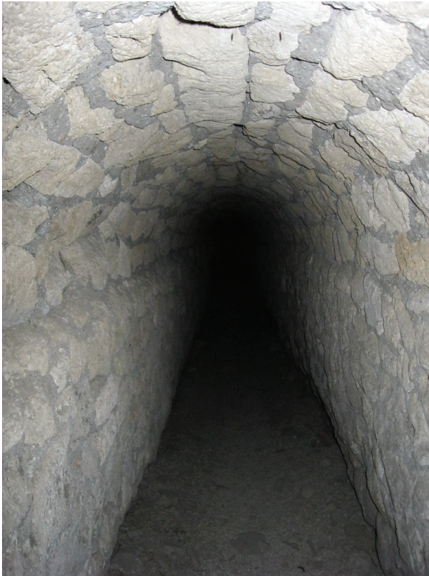
Figure 9: View inside the Altstadt sewer, facing north toward the Large Theater and farther to Stabian Baths.
