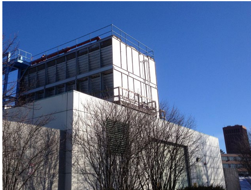
COOLING TOWER AT UMass
