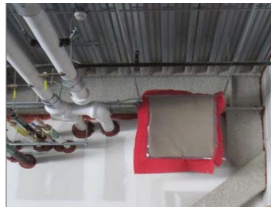
AIR HANDLERS MANAGE AIR QUALITY DURING CONSTRUCTION
