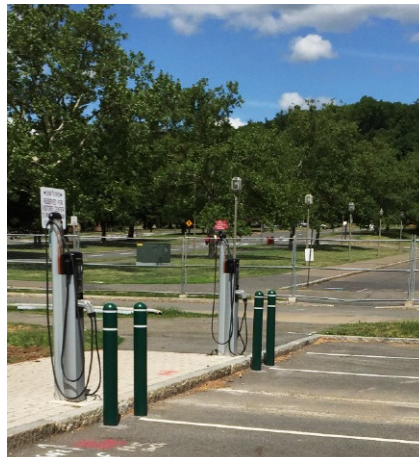
ELECTRIC VEHICLE CHARGING STATIONS, ROBHAM MEMORIAL VISTIOR CENTER
