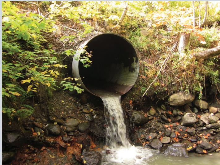
Old 7 foot pipe culvert. These types of culverts remain common in New England. In Vermont alone, 964 culverts were damaged, destroyed or blown-out during Tropical Storm Irene.
