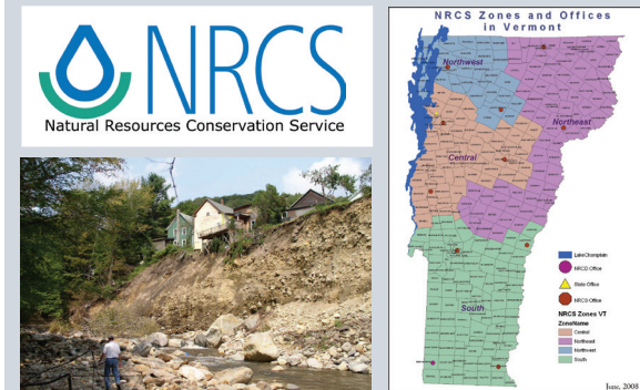
Tropical Storm Irene Damage, West Branch Deerfield River, Readsboro Vermont. NRCS VT Engineering Staff coordinated with NRCS employees from around the country to form teams who performed damage survey reports throughout the state. In 2011, NRCS VT investigated 193 damaged sites and determined 153 of them eligible for the Emergency Watershed Program. (Photo from NRCS, Conserving Natural Resources in Vermont, January 2012).
