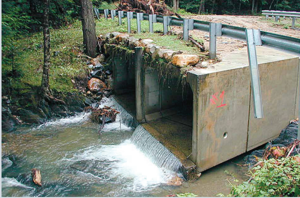
A double box culvert on Bronson Brook in Worthington, MA was long a barrier to fish due to a perched outlet, shallow water depths and excessive water velocities. It became clogged with debris during a large storm in August 2003, and failed catastrophically when it was overtopped with water and the fill around the culverts was eroded away. The stream dug a 14 ft. (4 m) wide rift between the road and the culverts.
