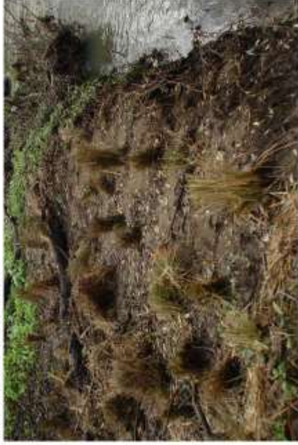
Station 2750: Levee Breach
