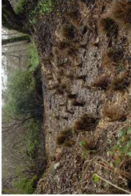
Station 2750: Levee Breach
