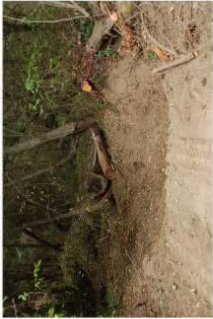
PP-13 facing northwest on 10/14/2014at excavated backwater pool (center) and wood complex (background). Access road is in foreground.
