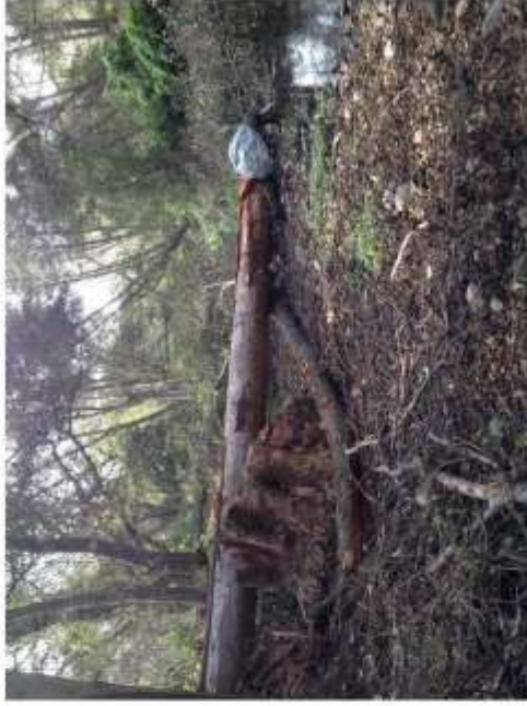
Facing downstream during construction on 10/9/2014. The excavator is placing a boulder on the streambed near the end of the redwood log
