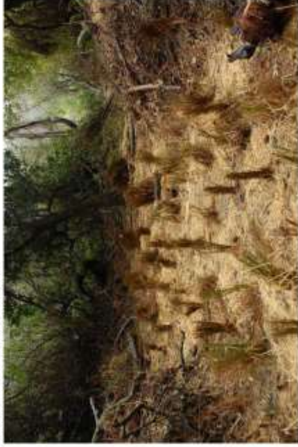
Station 2850: Levee Breach
