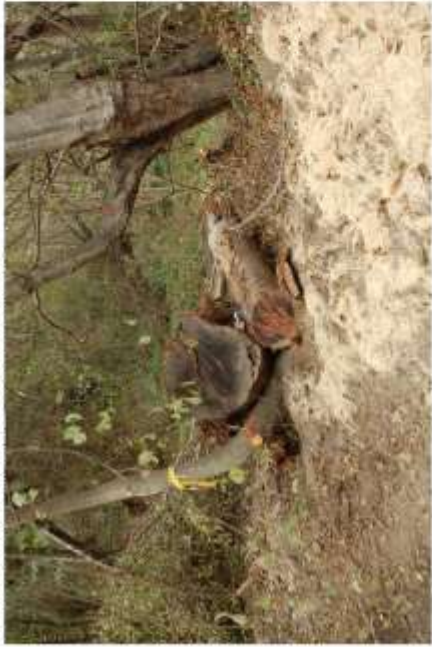
PP-13 facing northwest on 10/20/2014at backwater pool (foreground) and wood complex (center). Photo was taken following construction and mulch and before reveg.
