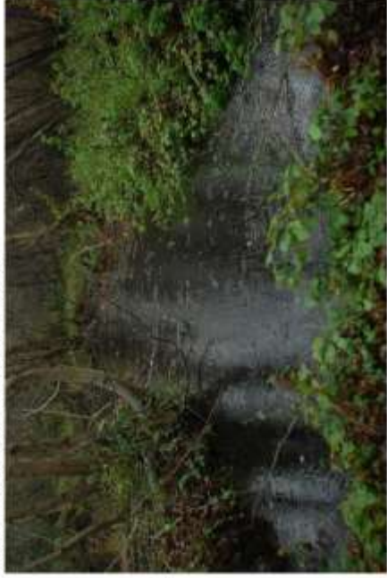
Station 1800: Scour Feature Connection
