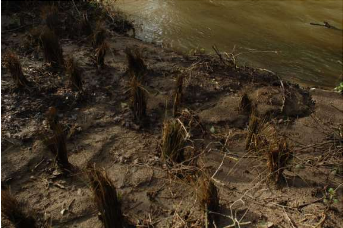
Figure 25. Rilling at the mouth of levee breach at 2000 on 12/18/2014
