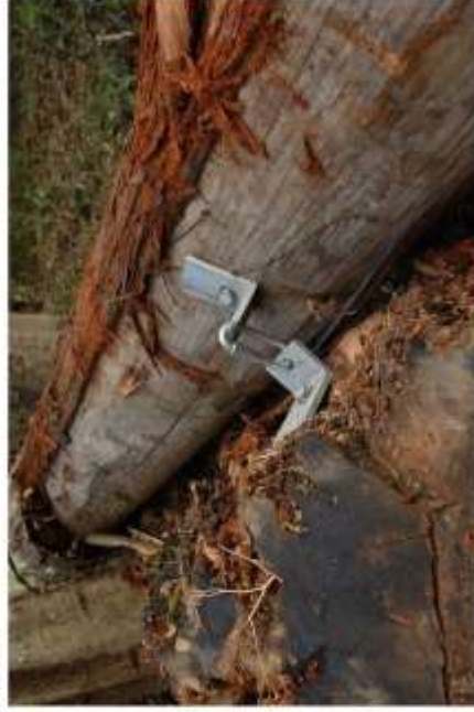
Photo taken on 12/3/2014 showing debris racking and slight movement of rootwad evident from visible upward displacement of quick link, visible at bottom right. Compare also to photo below taken on 10/20/2014 on the day the hardware was installed.
