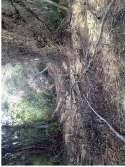
Station 1900: Levee Breach
