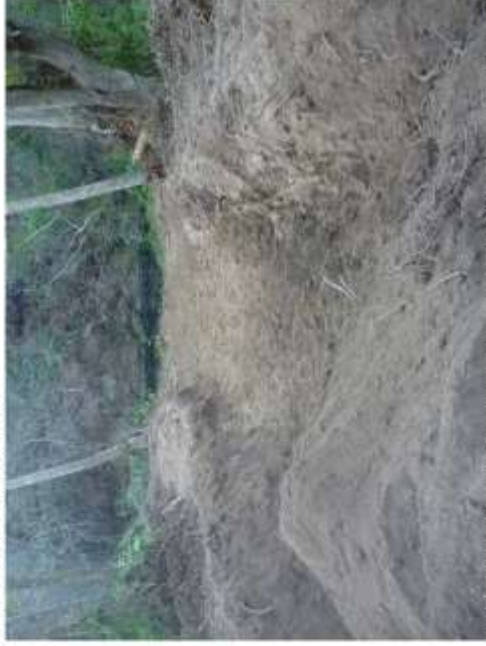
Station 2000: Levee Breach
