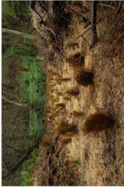
Station 2850: Levee Breach
