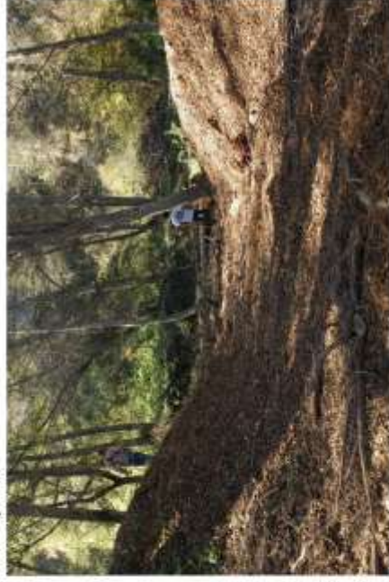
3) PP5 facing west at new breach opening on 10/14/2014. The stream channel is in the background.
