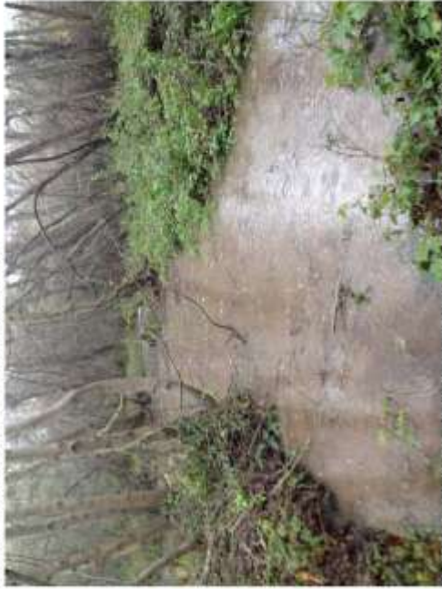
Station 1800: Scour Feature Connection
