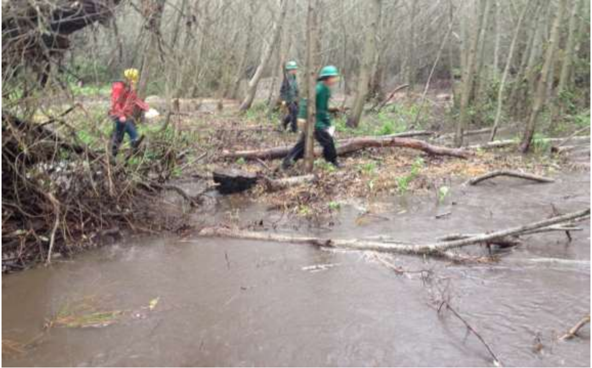
Figure 23. Looking NE on 12/11/2014 at breach at 1900 (foreground) and 2000 (background). Photo shows outflow through both breaches and floodplain inundation.
