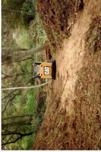
Station 2650: Levee Breach
