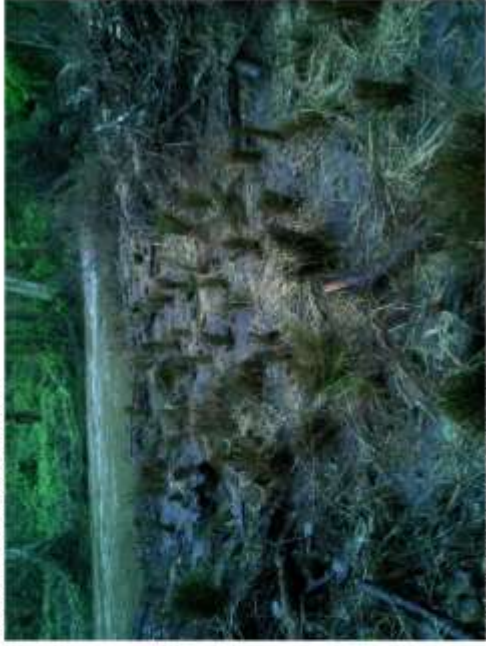
Station 2850: Levee Breach
