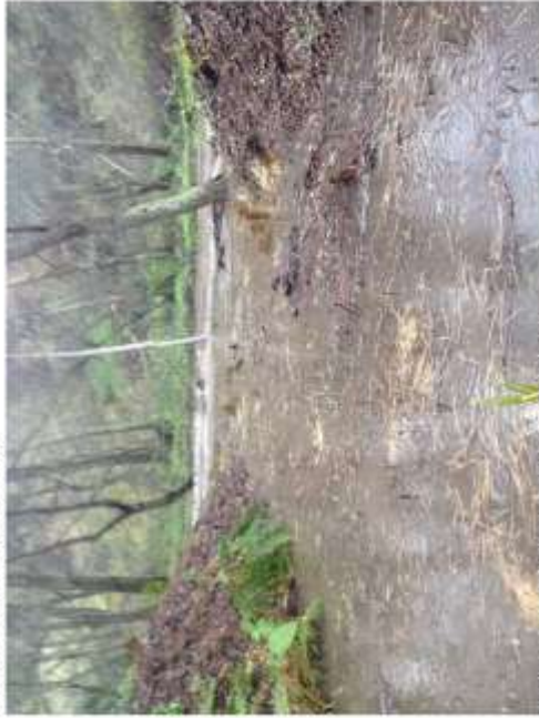
Station 2650: Levee Breach
