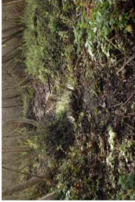
Station 1800: Scour Feature Connection
