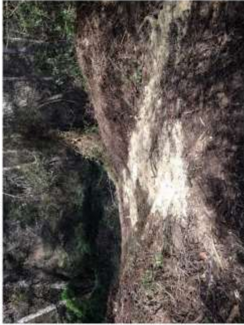
Station 2750: Levee Breach
