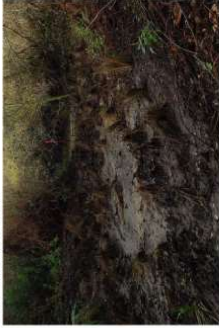
Station 1900: Levee Breach
