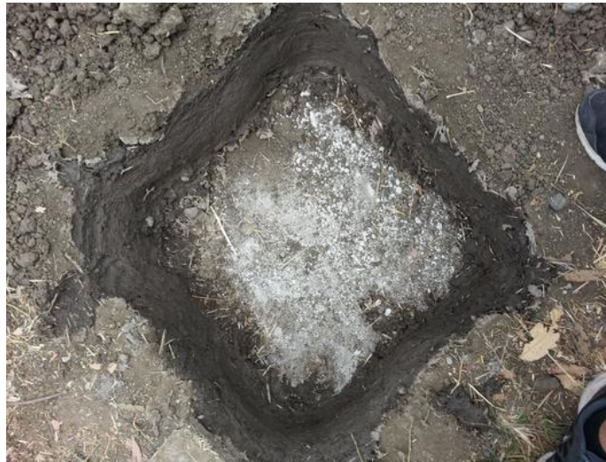
Figure 5.2: The first step was digging a hole which was approximately 3 ft. by 3 ft. and 12 inches deep. Basically, the hole should allow 10 inches of insulation on all sides of the pot, which is the minimum insulation for the desired thermal resistance. The sides of the hole were supported by mud/clay.
