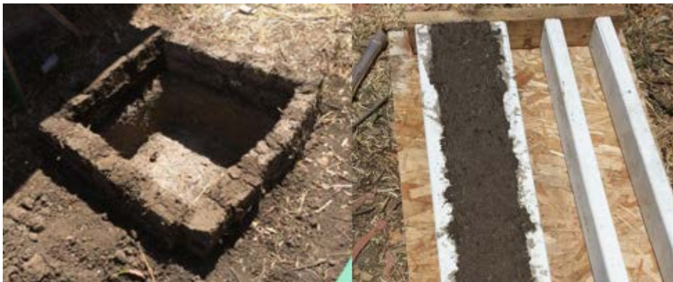
Figure 5.3: The dirt from the hole was used to make bricks by mixing mud and straw with a 1:1 ratio. We made a fixture made from plywood and 2x4 to compact and form the mixture into bricks. They were then cut using a saw to roughly 8 inch sections. The bricks were laid out and stacked around the hole so that the total height of the cooker was about 2 feet.
