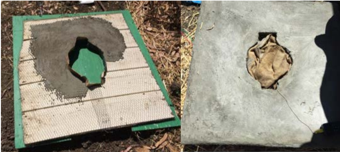
Figure 5.4: To make a countertop, we cut a hole in the middle of a piece of plywood and added two more holes to allow space for the hands to reach into the cooker. The top surface of the plywood was then covered with a wire mesh. A thin layer of cement and sand mixture was spread on the top surface of the counter. We smoothed and textured the top surface by spraying water and flattening the surface with a trowel.
