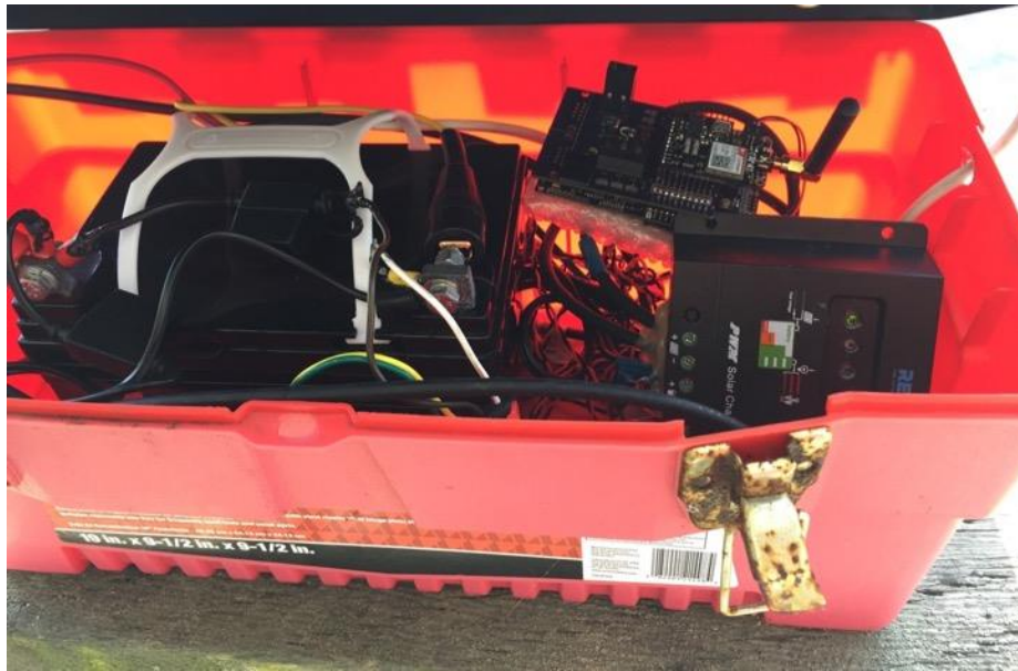
Figure 2: Remote Monitoring System with the Battery and Charger
