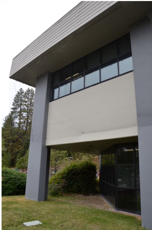
Figure 1: Chamfered corner at the southwest corner of the building
