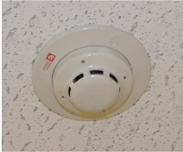
Figure 17: Photoelectric smoke detector connected to the main fire alarm system
