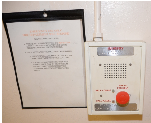
Figure 26: Emergency intercom system located at the top of the east stairwell
