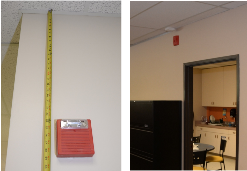
Figure 25: Notification devices installed too low, and too high in the building
