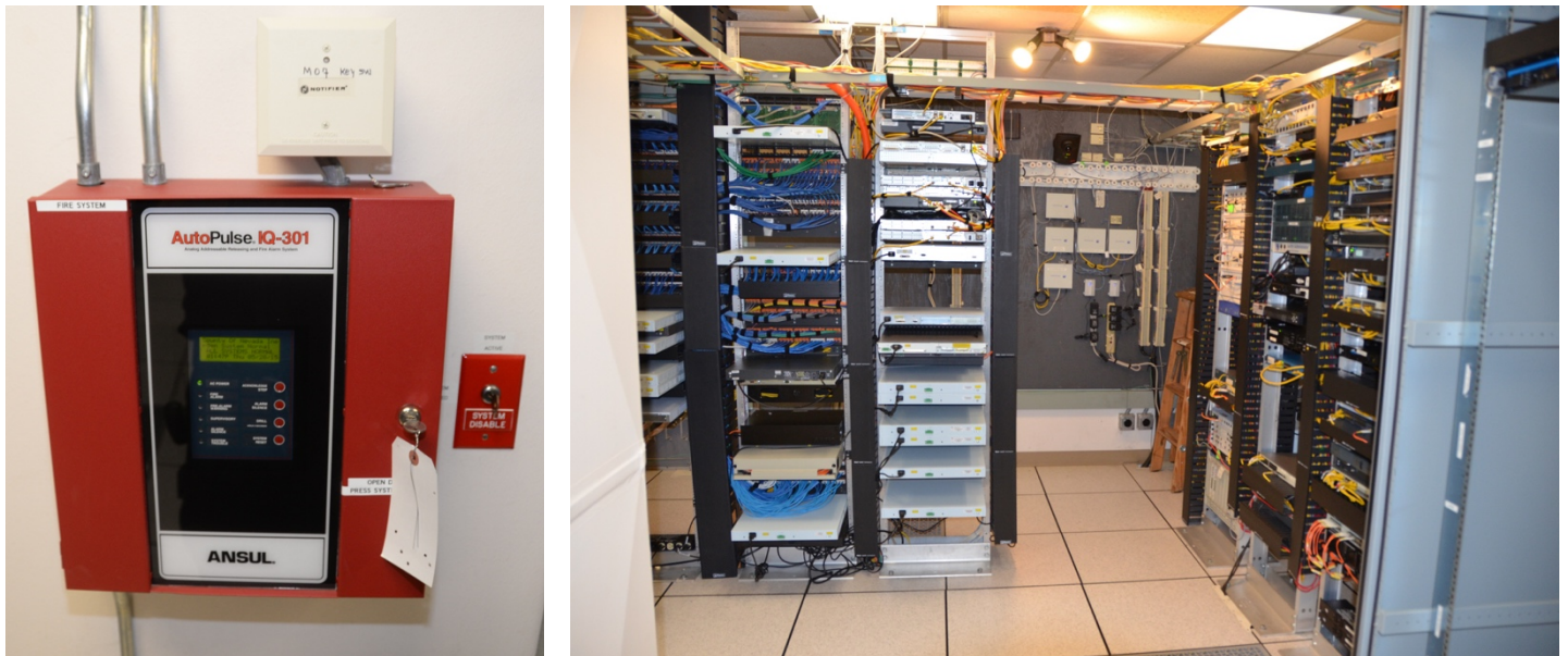
Figure 16: The secondary FACP located inside one of the server rooms
