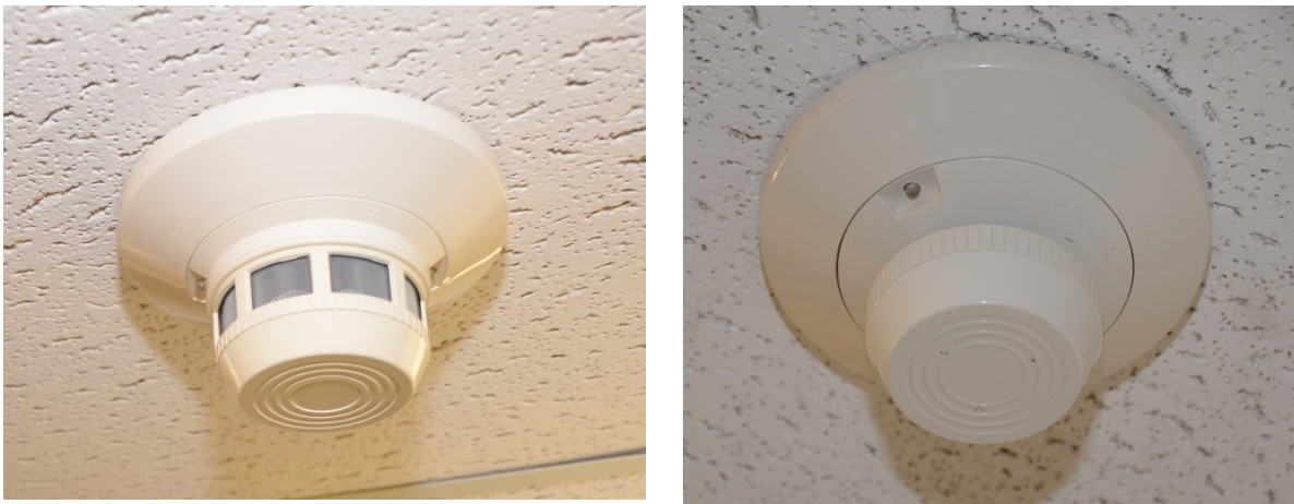
Figure 18: Photoelectric smoke detector on the left, Ionization smoke detector on the right connected to the secondary fire alarm system
