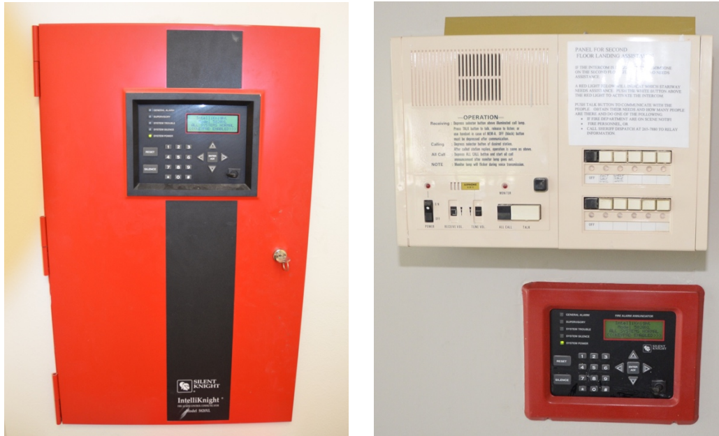
Figure 15: The main FACP, the remote annunciator, and the building's intercom system
