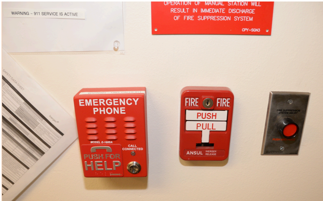
Figure 19: Emergency intercom system, manual pull station, abort switch in server room
