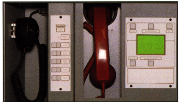
XLS1000 emergency paging and fire phone controls
