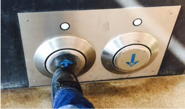
Figure 22. Foot activated elevator button
