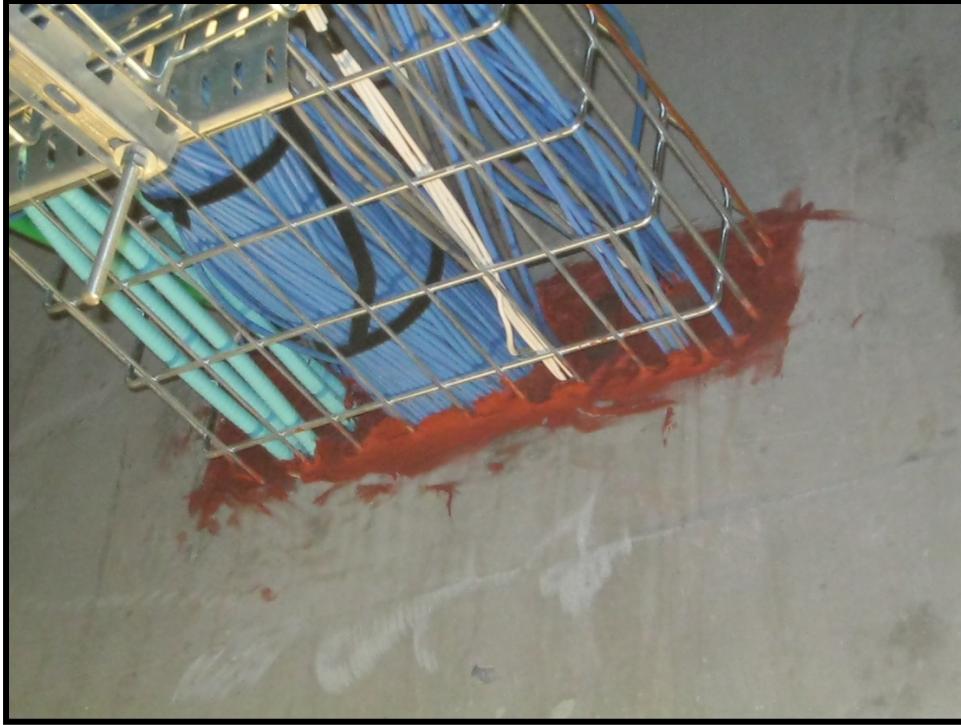
Figure 43: Typical cable tray wall penetration showing typical application of fire-stop material.
