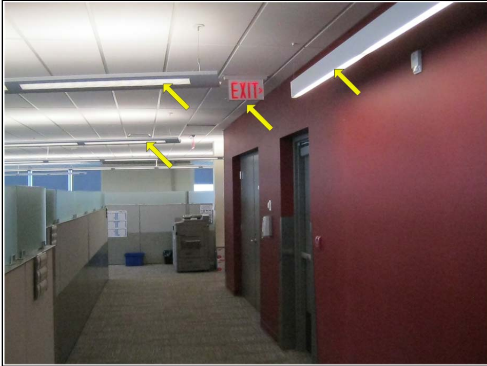
Figure 13: Emergency lighting and exit signs. The devices identified by the arrows remain illuminated following a main power loss by drawing on the building UPS. Only the end lamps above the corridor are on the UPS.
