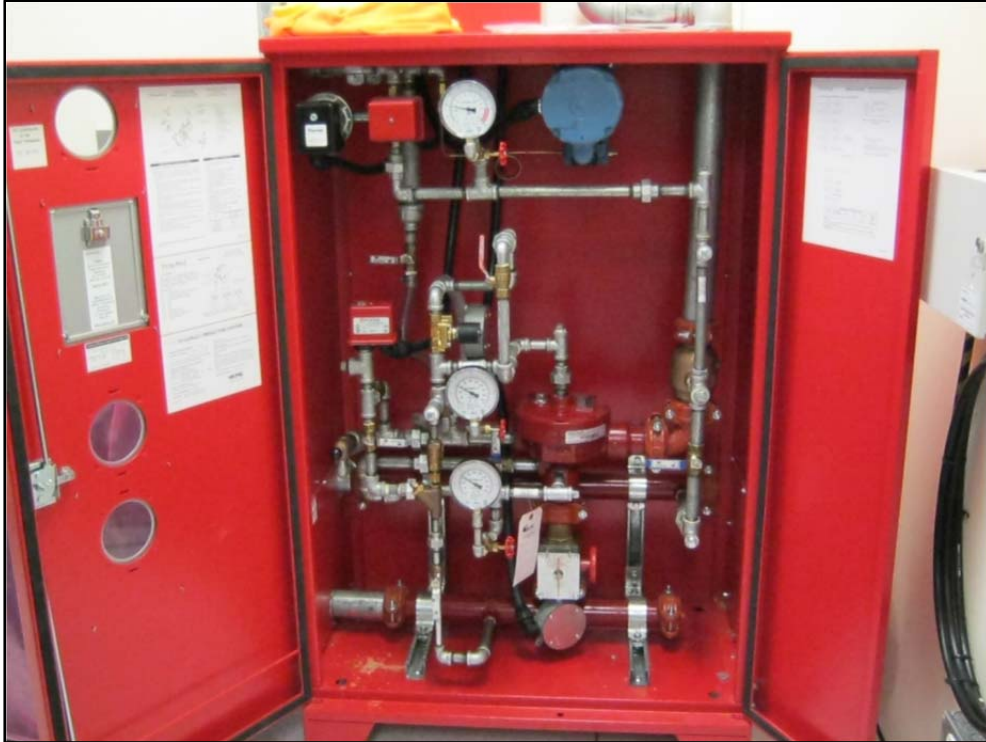
Figure 16: Preaction deluge valve located in the POP room
