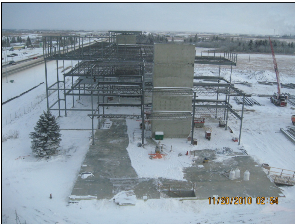
Figure 11: Egress from the basement is via the West Exit Stairway Enclosure or the exit stairs that can be seen passing through the basement roof slab in the foreground.
