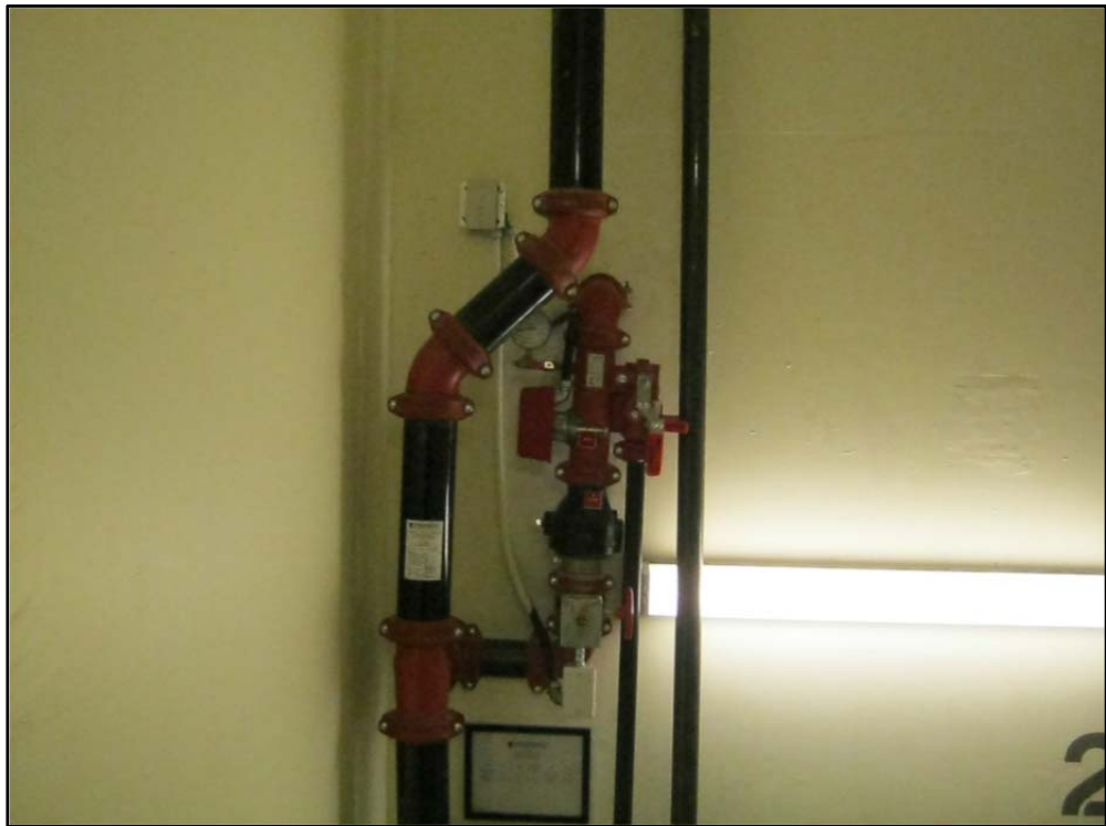
Figure 27: A typical floor control valve arrangement
