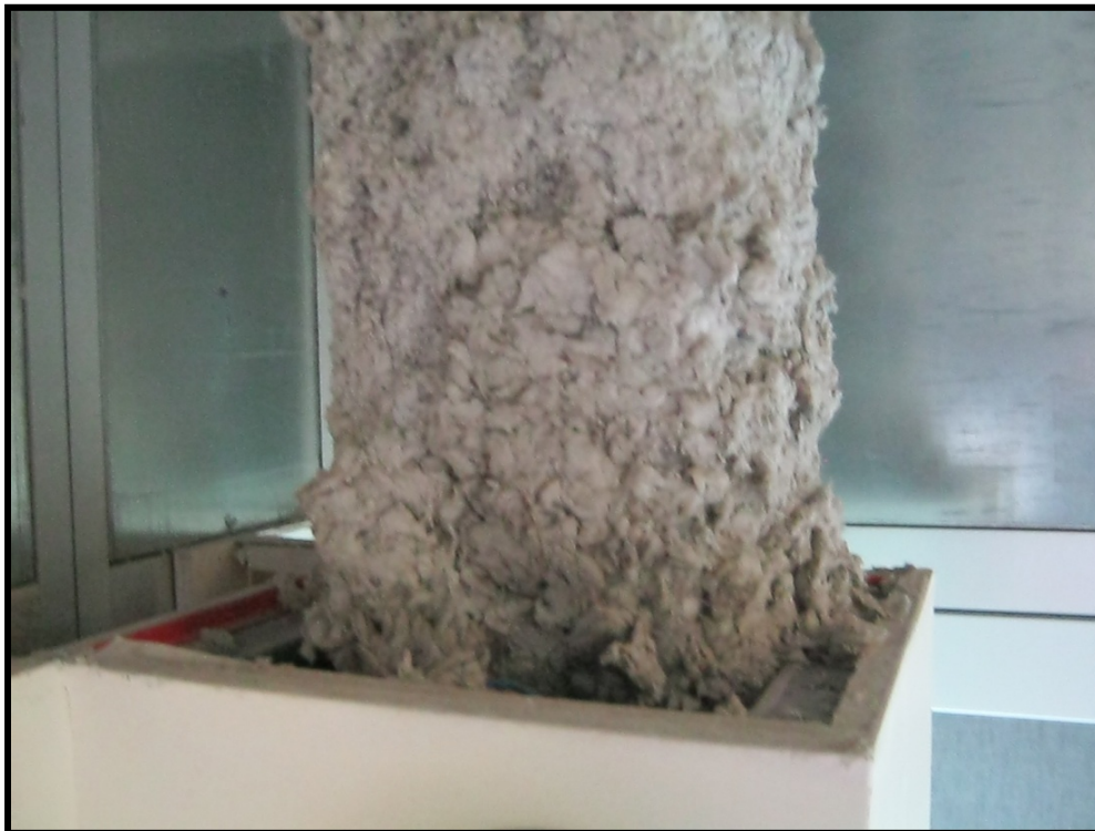
Figure 37: Fire proofing visible above the gypsum wall board applied for esthetic purposes.
