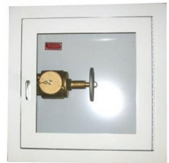
Figure 34: Fire Hose Valve Cabinet
