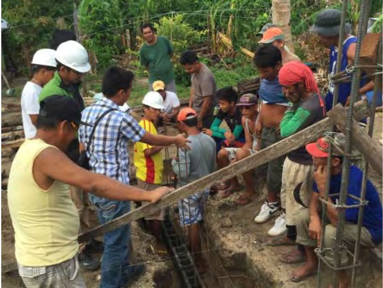
Figure 9: In this image the locals are observing how rebar should be tied in columns. On the right side of the picture there is column steelwork that is all tied up and ready for concrete. notice that the column steelwork has been leveled out and supported with wood cross braces in preparation for the concrete pour.
