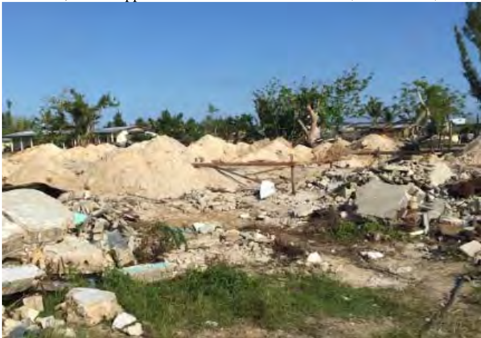
Figure 12: This image displays the rubble that had to be cleared from the site location for the ESSU Construction Training Facility in Guiuan, the Philippines. (South Side)
