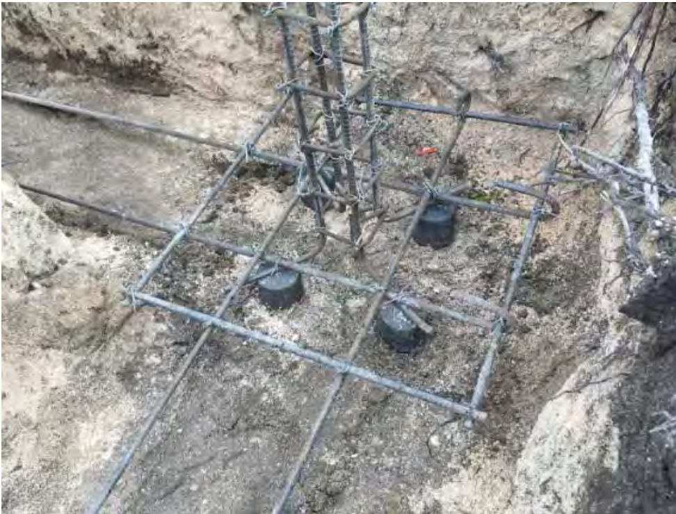
Figure 6: This rebar is for the column foundation which will be poured after the CMU is placed on the sides as seen in some of the following figures.
