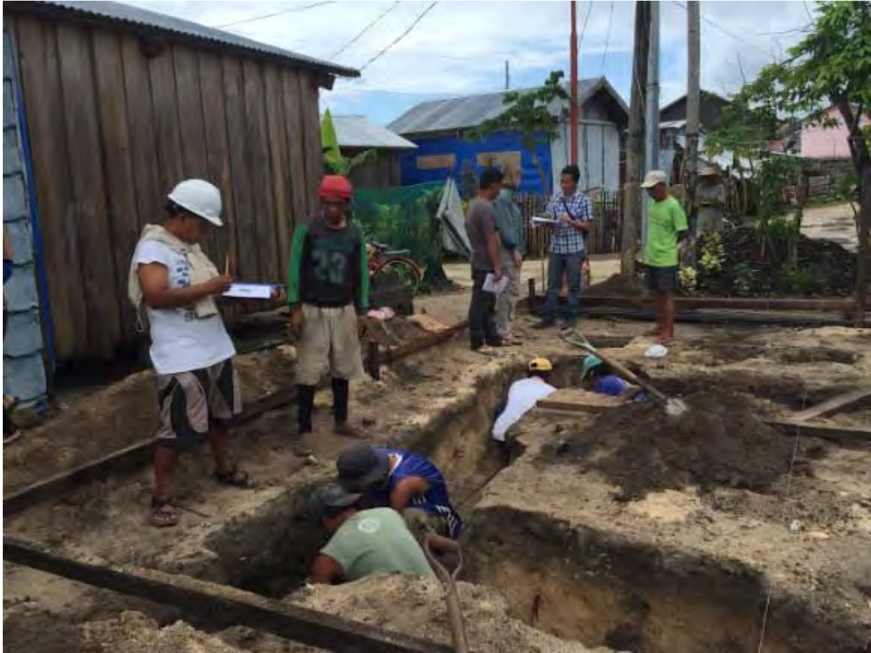
Figure 8: This image shows the initial digging of the foundation trenches. Pay close attention to the small work area of the work station as it plays a huge roll in the design of the general site layout.
