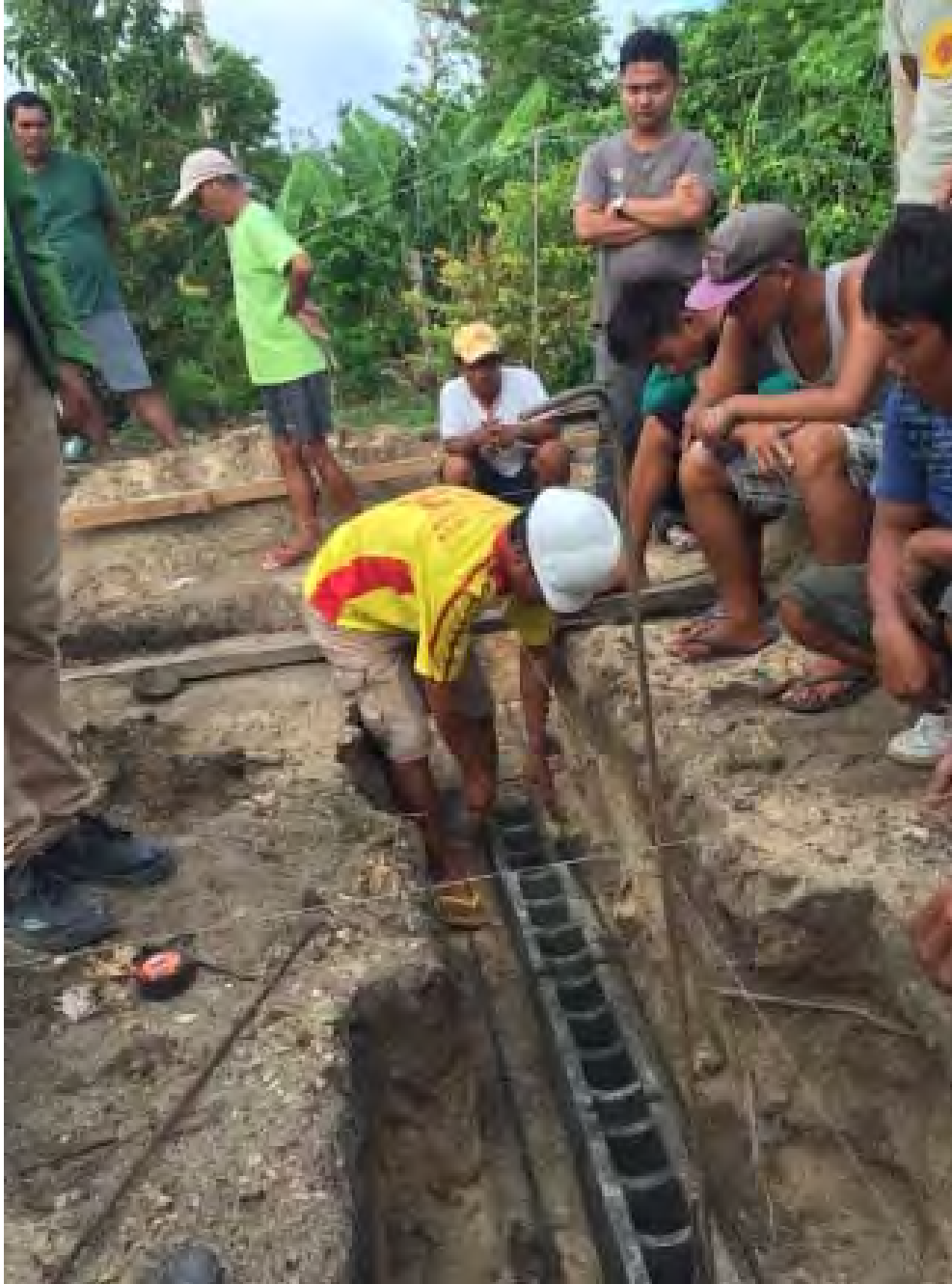
Figure 7: Local Pilipino mason places foundation CMU blocks and is getting ready to place the horizontal rebar above the CMU. The horizontal rebar can be seen laying besides the CMU.
