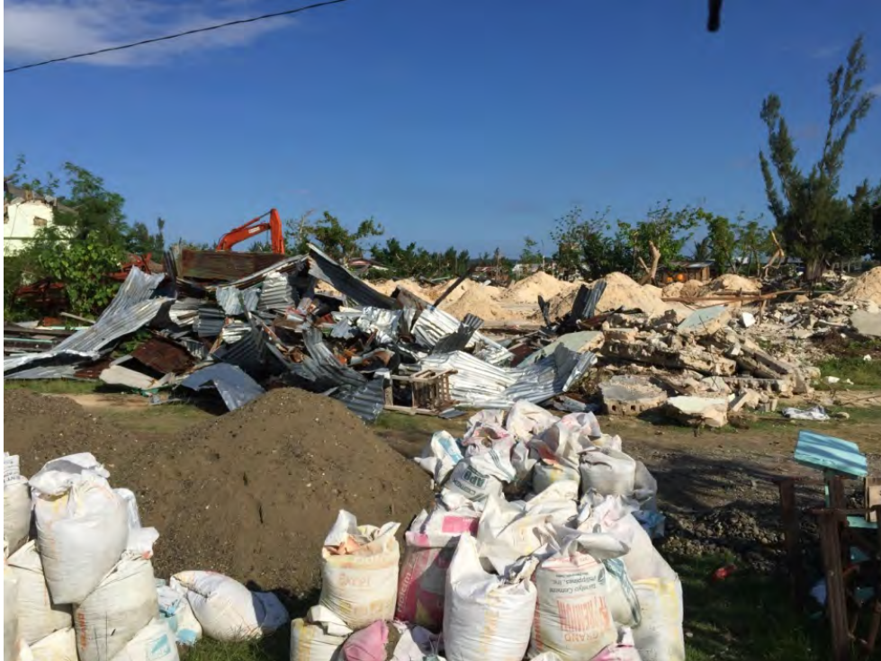
Figure 11: This image displays the rubble that had to be cleared from the site location for the ESSU Construction Training Facility in Guiuan, the Philippines. Mini Excavator in the back (Northeast Corner)
