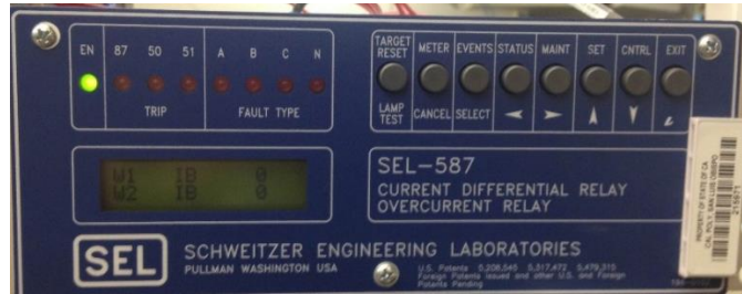
FIGURE 7 FRONT PANEL FOR SEL 587. DISPLAYS BOTH NORMAL OPERATION AND POTENTIAL FAULT CONDITIONS.
