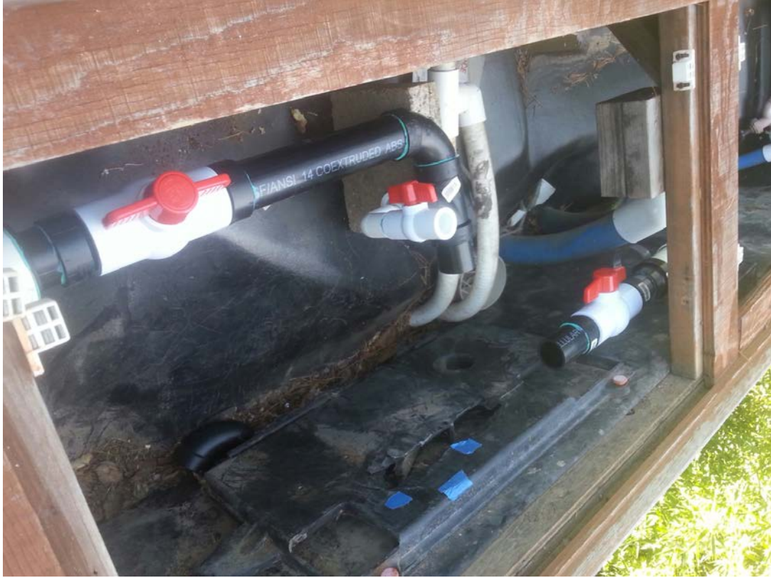
Figure 4.3: Pre-Pump-Installation Plumbing Connections
