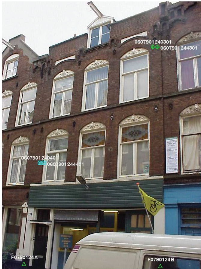
Fig. 16. (Color) Façade with monitoring points for Govert Flinckstraat 124 (Ceintuurbaan) (reproduced by permission of Frank Kaalberg, Witteveen+Bos)
