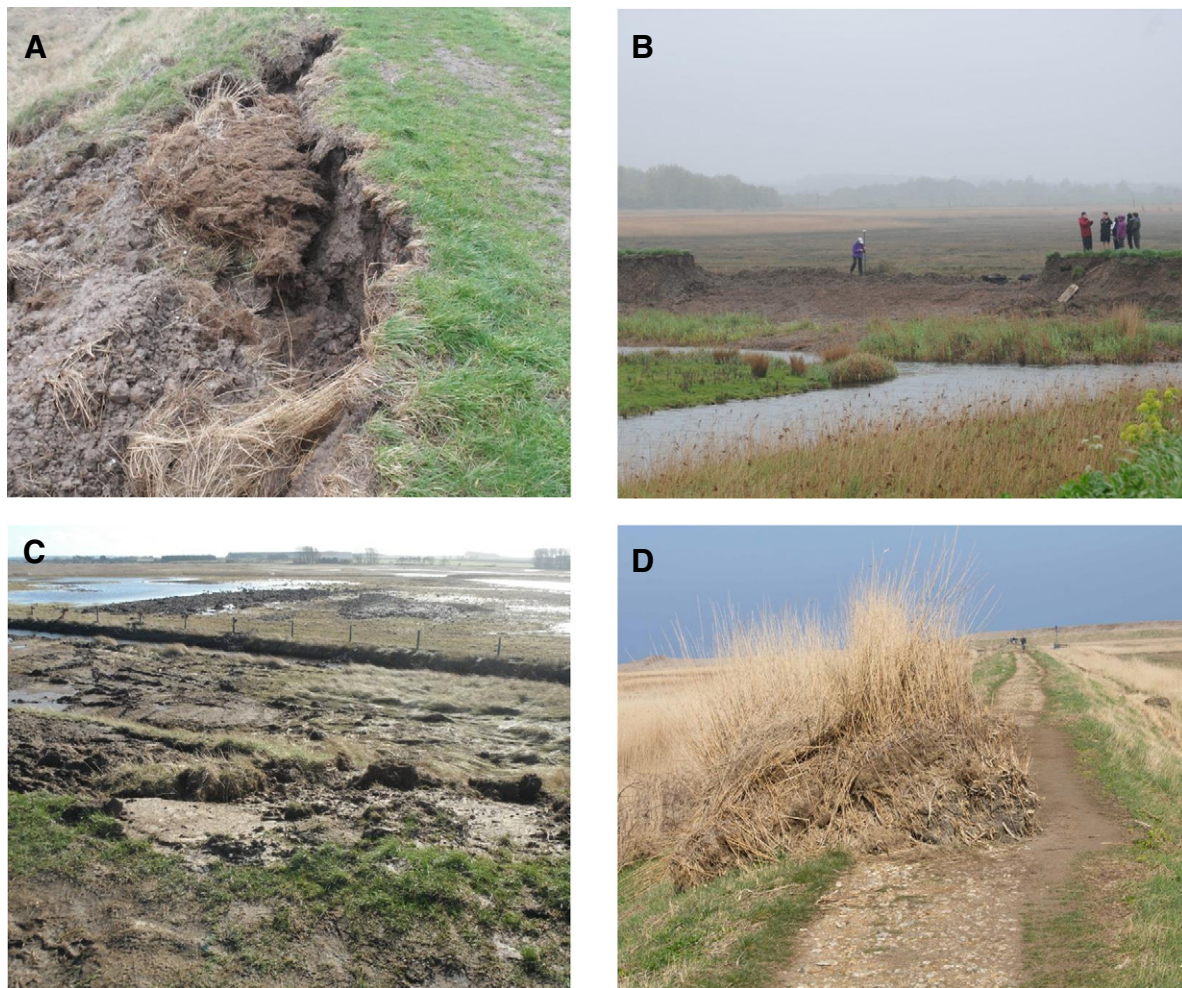
Fig. 14. Failure mechanisms in earthen banks, North Norfolk. A) Vertical fissures in landward face following overtopping, Burnham Norton seawall (reclaimed marsh to left); B) breach in earthen bank, west margin of Brancaster West Marsh managed realignment, looking west to exterior saltmarsh. Note vertical landward faces on either side of breach; C) arcuate mud boulder debris field beyond boundary fence inside breach (seen lower left) at Burnham Deepdale; D) reeds on plucked wetland block, Clay seawall. Photographs: A) T Spencer 14 February 2014; B) A Martin 25 March 2014; C) T Spencer 16 February 2014; D) G Fuller 9 March 2014.
