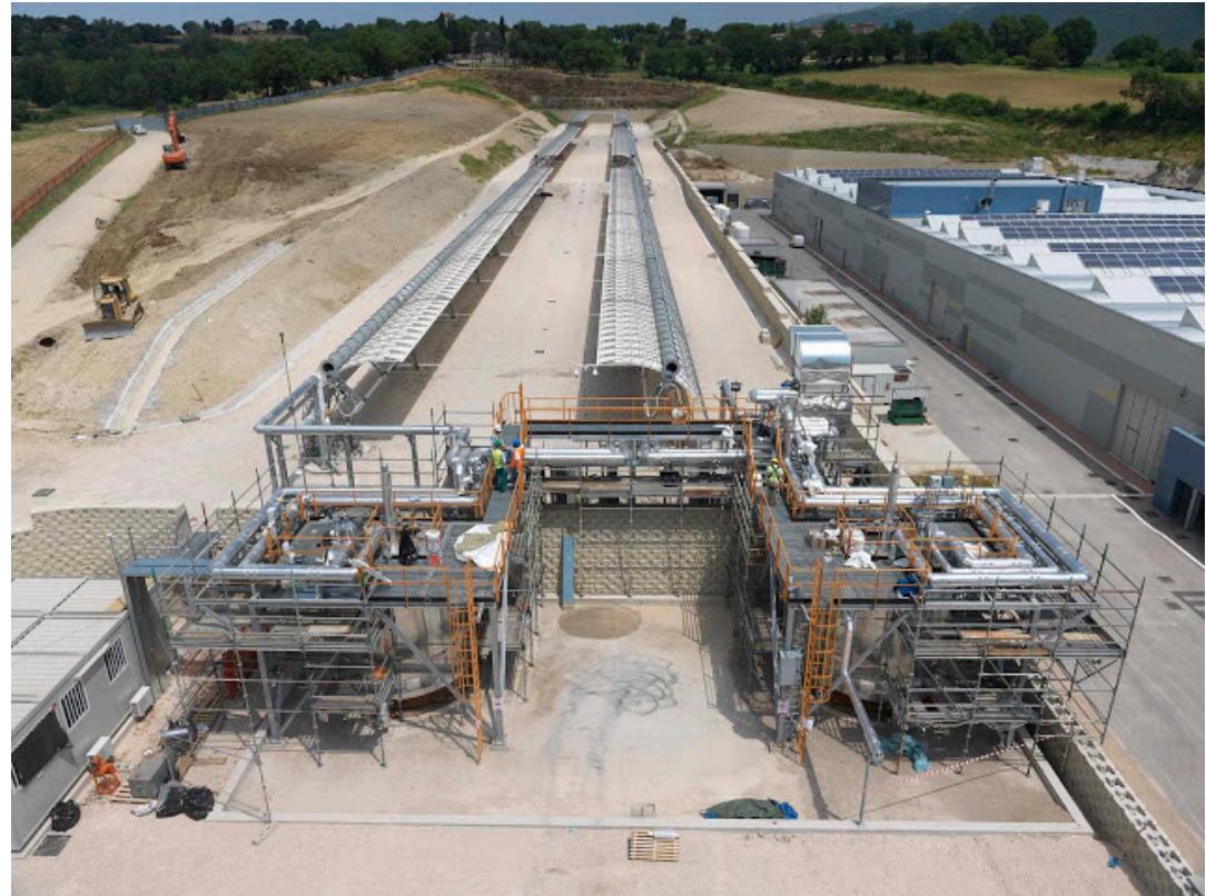
Source: Archimede Solar Energy
