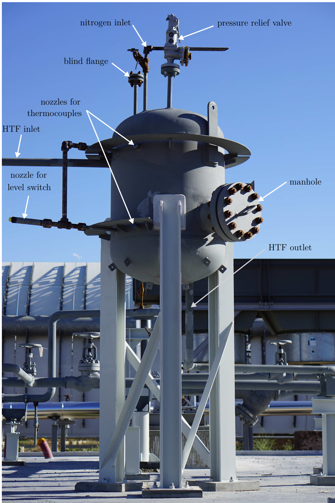
Figure E.3: Photo of the expansion vessel
