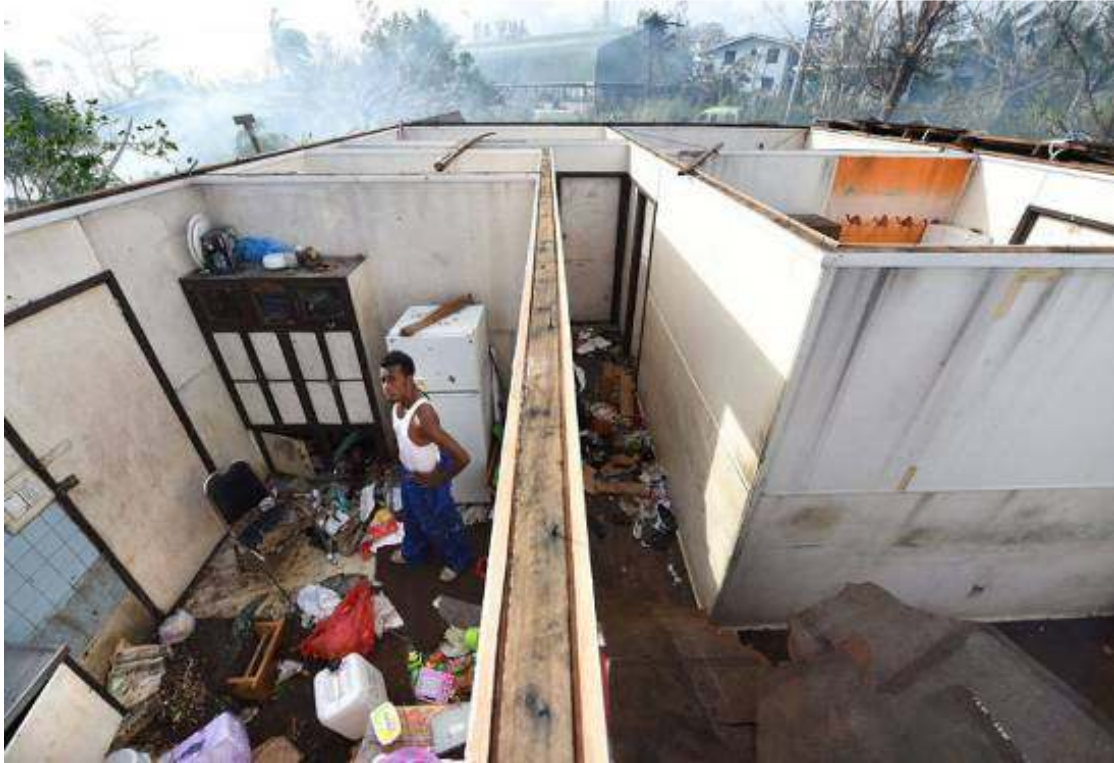
Fig. 4. Roof for the collection of rainwater being blown by the cyclone PAM
