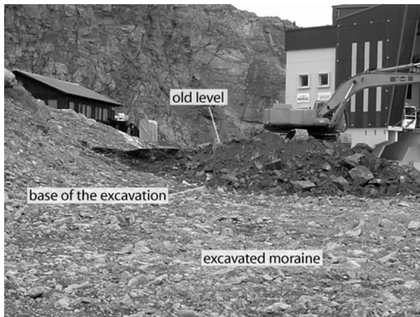
Fig. 3. Excavation works carried out in October 2006 to the south of the cable car station, on the road leading to the glacier.
