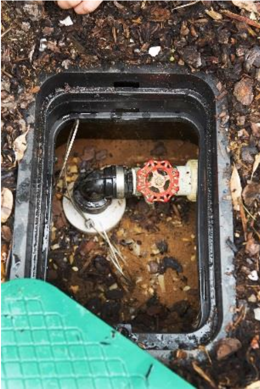
6C: Groundwater bore.
