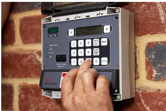
6A(ii): Irrigation system – controller.
