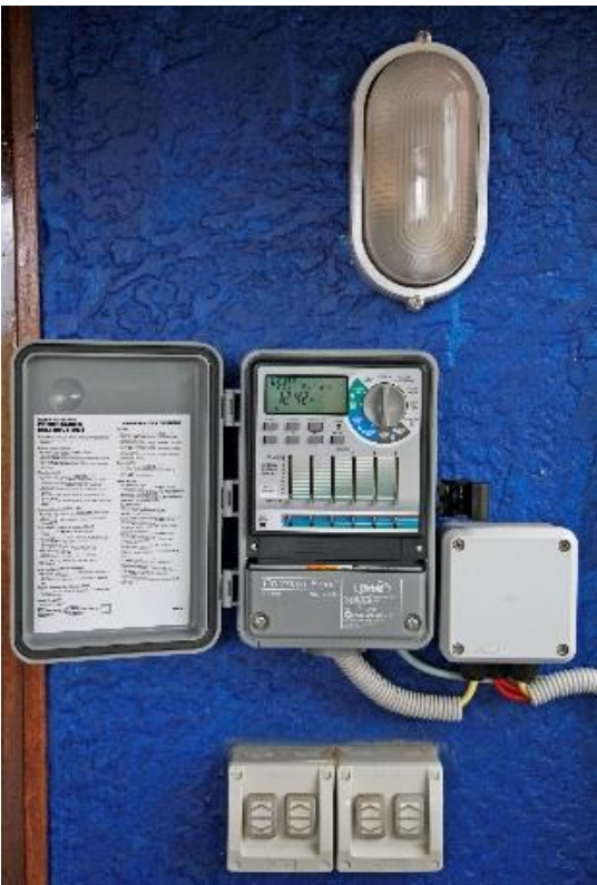
6A(ii): Irrigation system – controller.
