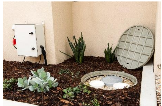
6B(i): Greywater system – access covers to sumps and submersible pump.
