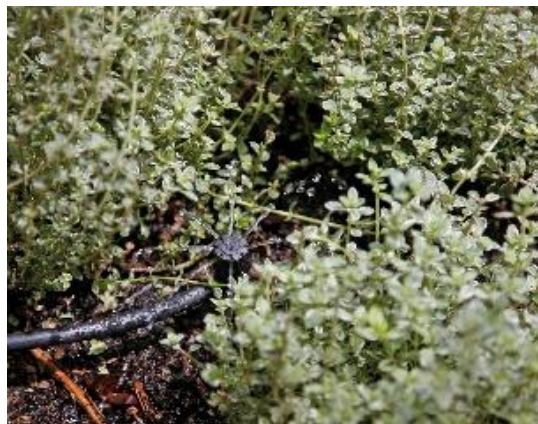
6A(v): Irrigation system – pot drippers.
