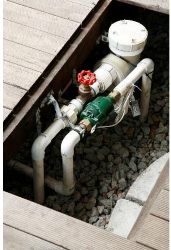
6B(iii): Greywater system – filter and meter.
