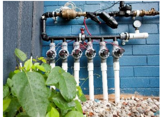
6A(i): Irrigation system – valve manifold.
