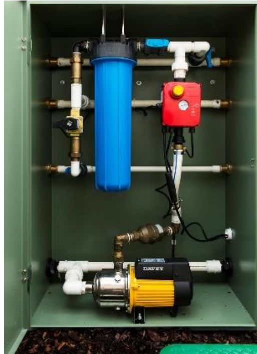
6D(iii): Rainwater system – pump and mains water backup valve.
