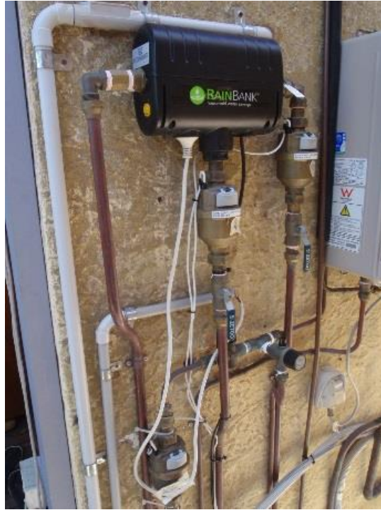
6C(iii): Rainwater system – mains water backup valve.
