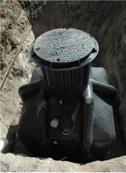
6C(i): Rainwater system - tank.
