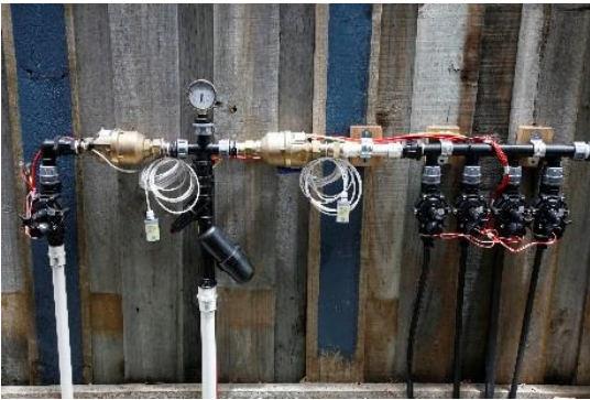
6A(i): Irrigation system – valve manifold.
