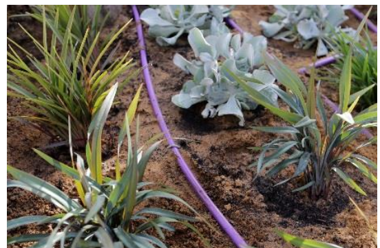
6B(ii): Greywater system – Dripline.
