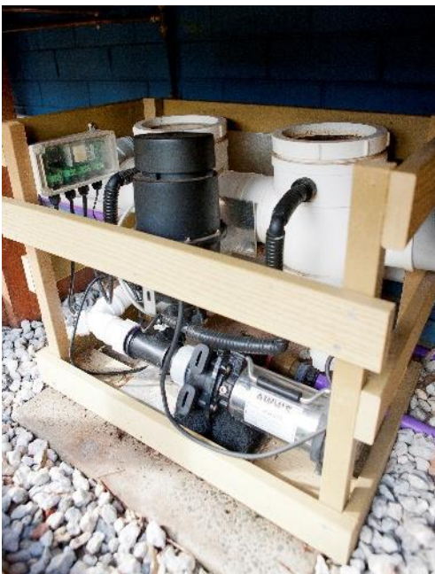
6B(ii): Greywater system – collection sumps, pump and blower.
