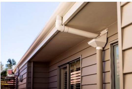
6D(ii): Rainwater system – rain head with leaf screens.
