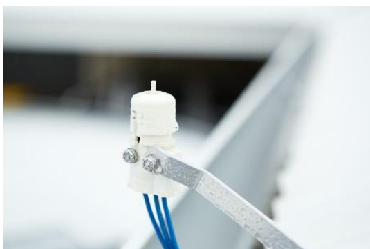
6A(iii): Irrigation system – rain shutoff switch.
