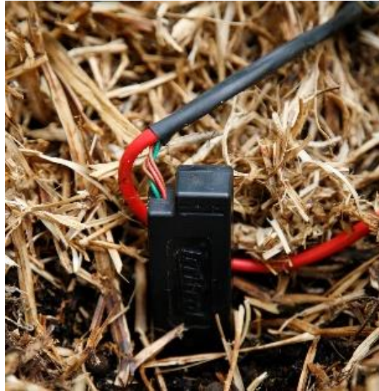
6A(iii): Irrigation system – soil moisture sensor.
