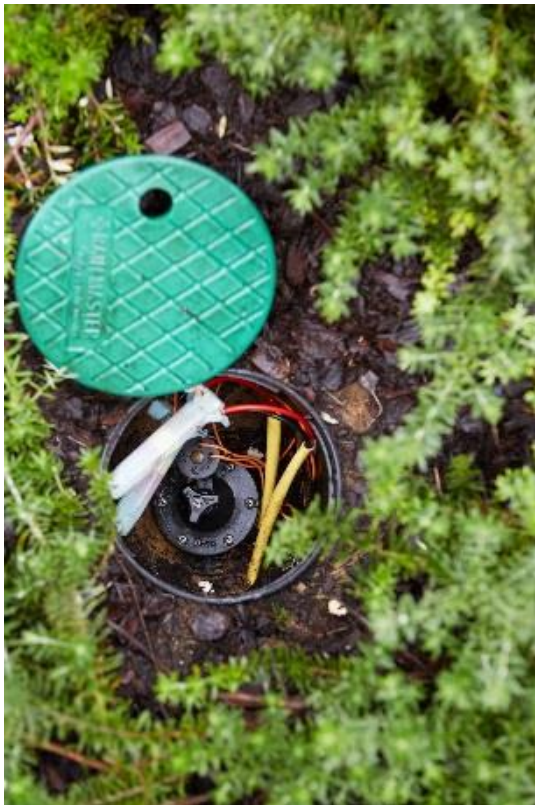
6A(i): Irrigation system – solenoid valves.
