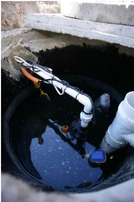
6B(ii): Greywater system – pump out tank.
