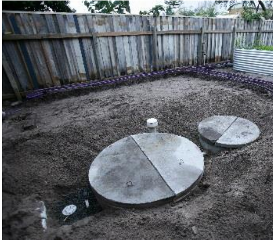
6B(i): Greywater system – settlement and pump out tanks.
