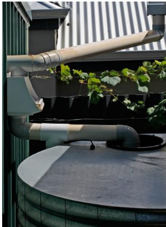
6C(ii): Rainwater system – rain heads with leaf screen.
