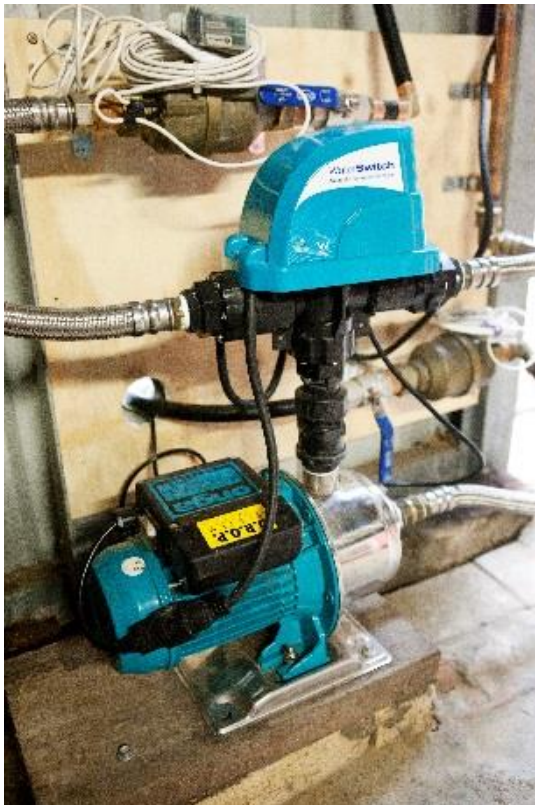
6C(iii): Rainwater system – pump and mains water backup valve.
