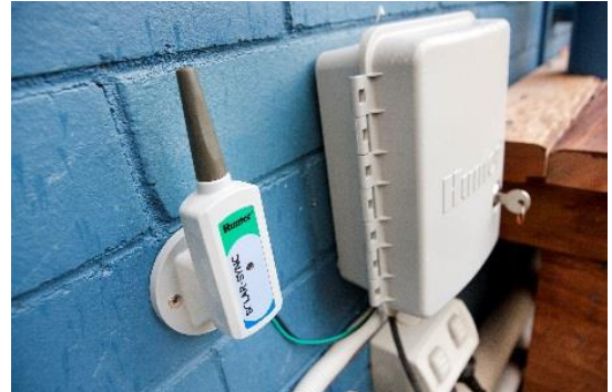
6A(ii): Irrigation system – controller.
