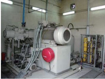
Figure 3. LMF natural gas compressor utilized in the station.
