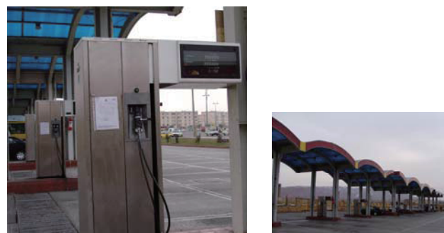
Figure. 1. CNG station for buses and cars in Maragheh , north-west of Iran
