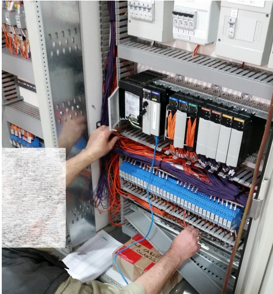
Figure 17: (Clampton, 2015) – Technician tracing cable for loose connections, electrical drawing is consistent or tags labelled on the wire are correct.
