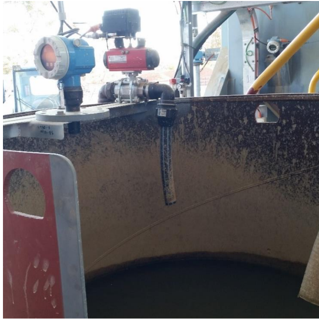
Figure 20: (Clampton, Site - Commission, 2015) – Tailings vat showing sump water output and ultrasonic level sensor.
