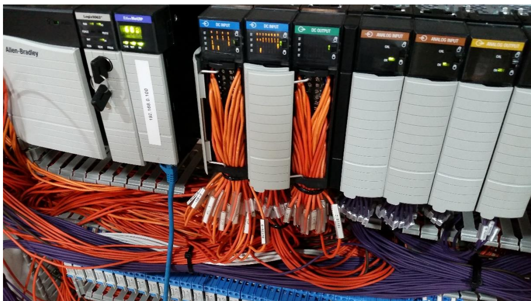
Figure 15: (Clampton, 2015) – the Allen-Bradley PLC rack showing all card attachments DC and Analogue I/O cards, communication card (Ethernet) and logix5000 processor.
