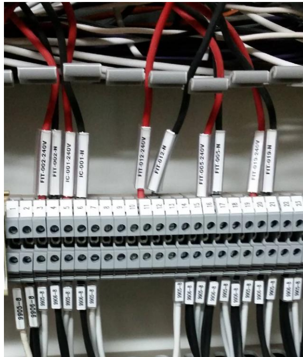
Figure 21: (Clampton, Site - Commission, 2015) – After reading the control philosophy and wiring diagram the spare I/O was found in the MCC.
