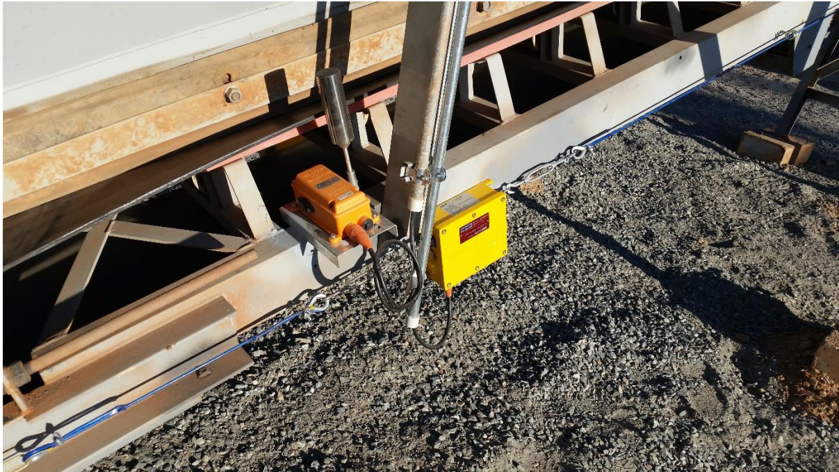
Figure 29: (Clampton, Site - Commission, 2015) – Tilt switch and lanyard emergency stops for conveyor belt.
