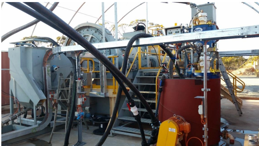
Figure 19: (Clampton, Site - Commission, 2015) – System as found first day, still in process of installation. Throughout commissioning the control team will be updated on changes or completion of systems so that they can be tested for compatibility with the control system.
