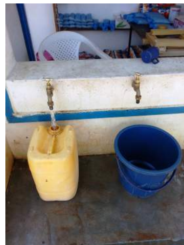
Figure 8: Water kiosk providing water to households in Ribáuè.
