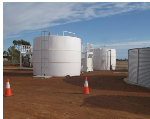
Figure 4.33: Waste water aeration and settling tanks
