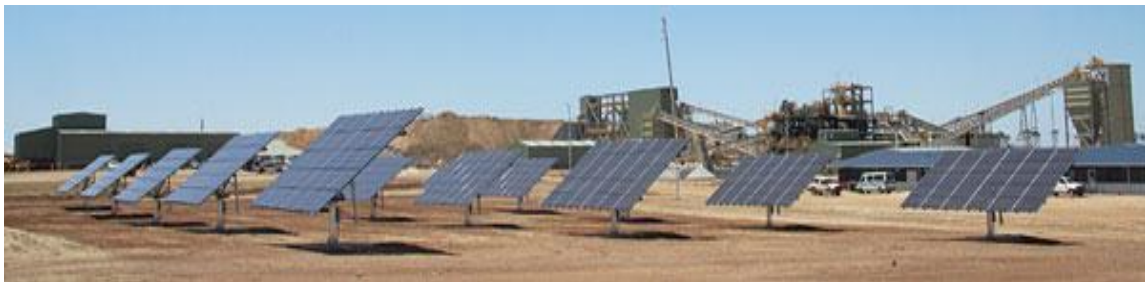
Figure 2.10 Solar tracking PV array at Mt Cattlin
