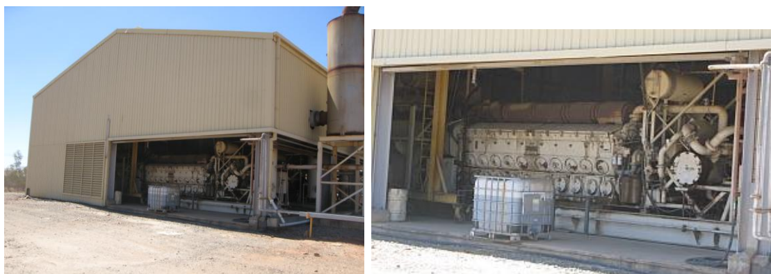
Figure 3.17: Diesel power generators at MMG mine
