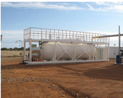
Figure 4.32: Waste water primary receiver tank for anaerobic treatment
