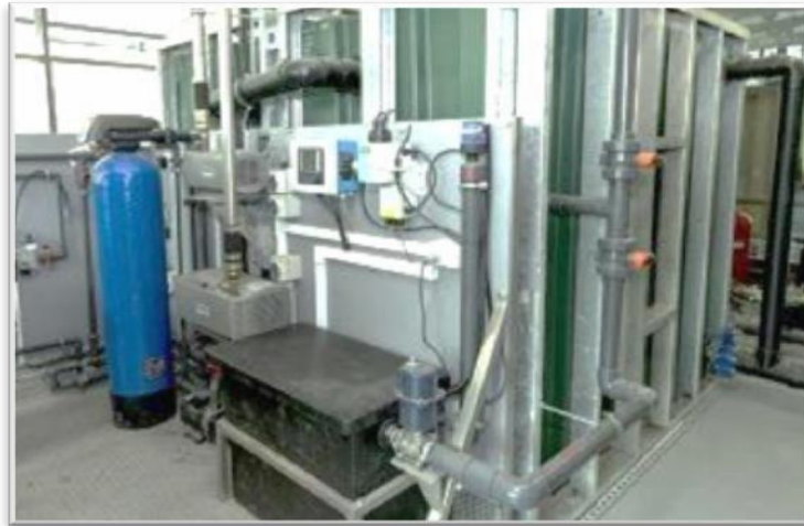
Figure 5. Exposed blackwater treatment system.
