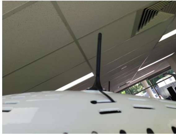
Figure 9: A half dipole whip antenna on top of a luminaire with coaxial cable
