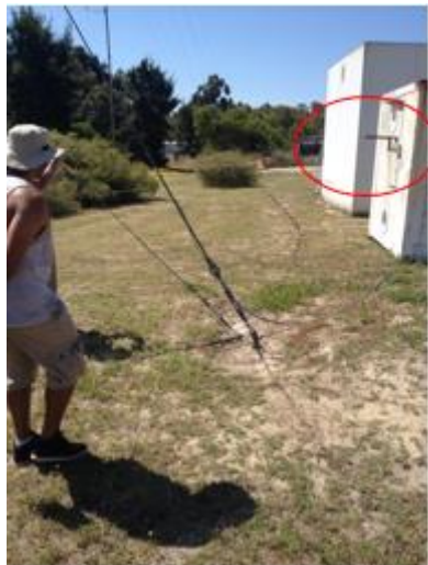
Exposed Metal Hazard
