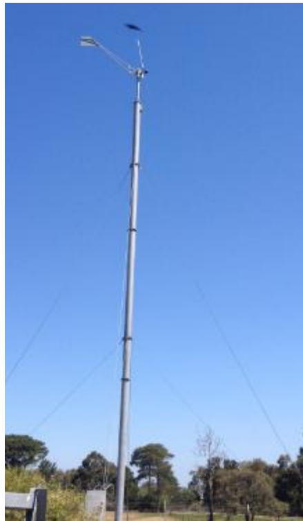
Figure 15- FP 1.4KW Wind Turbine
