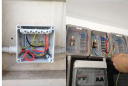
Figure 12-Wiring to Controller Box
