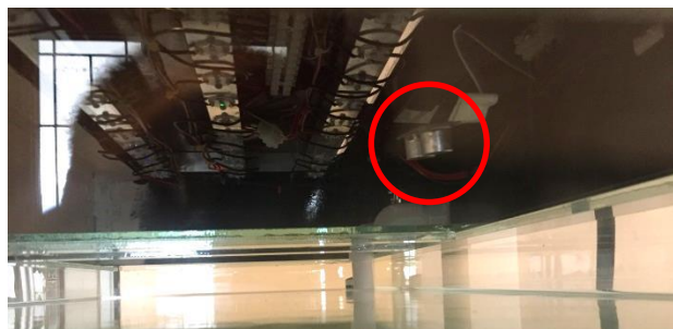
Figure 7-1 – Ultrasonic Sensor Over Main Tank.
