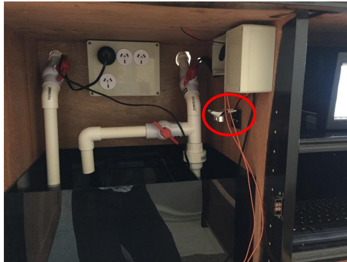
Figure 7-3 – Ultrasonic Sensor Over Sump Tank.
