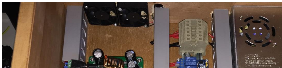
Figure 7-5 – Exhaust Fans for Cooling the Electrical Draw.
