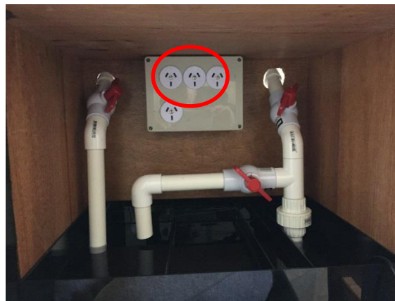
Figure 7-2 – Return Pump Controlled 240V Outlet.
