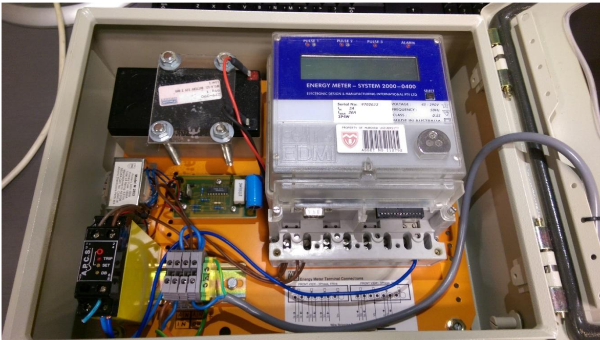
Figure 3 – Energy Meter – System 2000 - 0400
