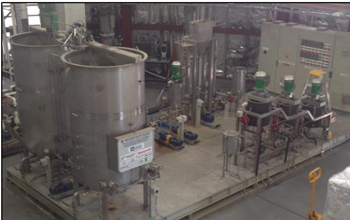
Figure 1: Murdoch University Pilot Plant
