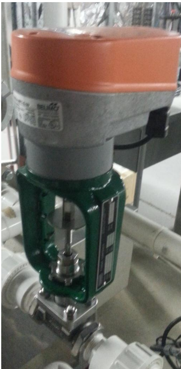
Figure 12- electric flow valve installed in the UWS
