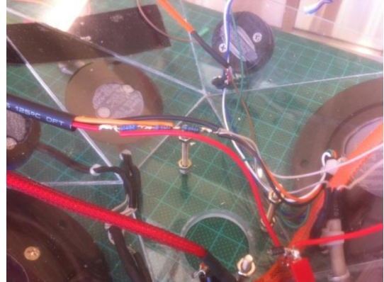
Figure 24, The Battery Voltage Divider
