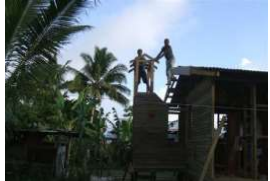
Figure 2.2.3k. The kitchen extension and tall chimney (right) designed, made and tested to best available village skilled artisans and technology for Eroni and Susannah .
