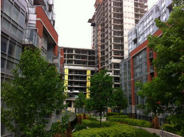
Above: Westside Lofts by Landmark Developments at 150 Sudbury St. Photo by author
