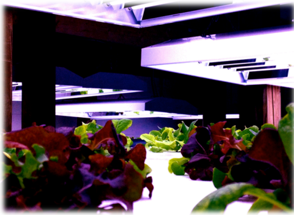
T5 Florescent lights used at the upStream Aquaponics facility in Newmarket, Ontario.
