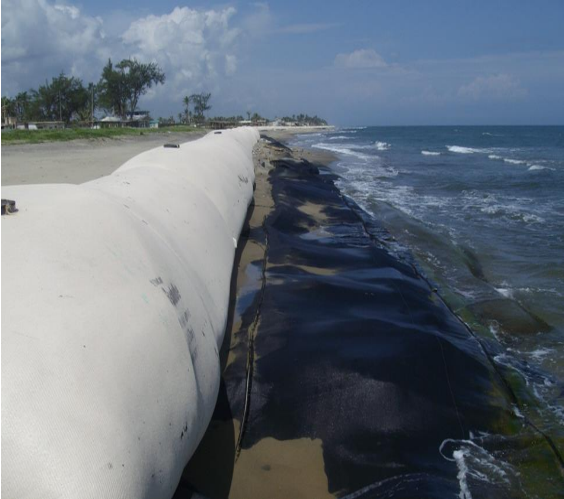
Figure 35. Coastal infrastructure – geotubes - to protect the coast from erosion, These geotubes are replacing rubber tubes that were previously built in this area but that have been destroyed by the effects of the sea and also (as it was explained in some interviews) by people.
