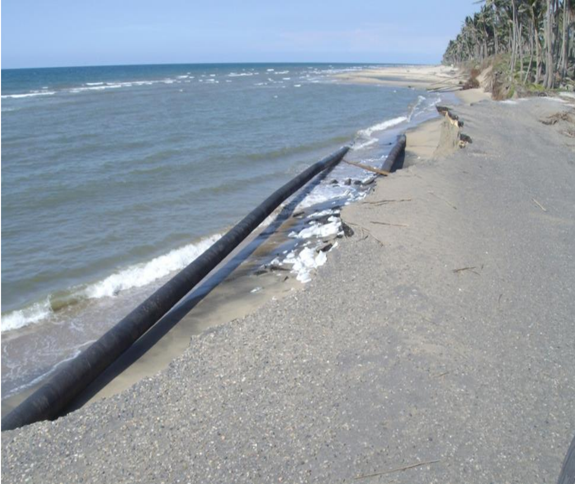
Figure 32. Coastal erosion impacts on oil infrastructure (pipelines).
