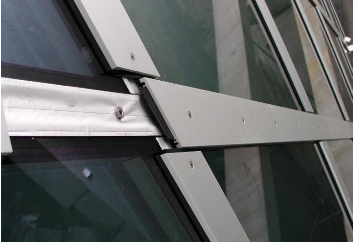
Figure A.23. Aluminum tape, primary water proofing barrier (Courtesy of © Marc Simmons, 2015)
