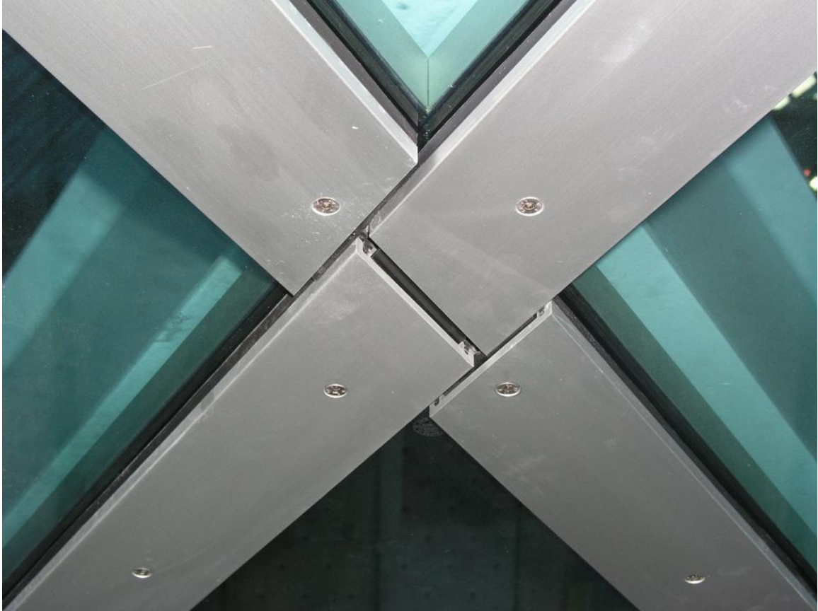
Figure A.8. Façade face cap holding the glass (Courtesy of © Marc Simmons, 2015)
