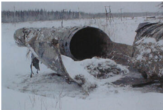
Figure 13: Photograph of pipe fracture resulting from stress corrosion cracking near a field weld[10]
