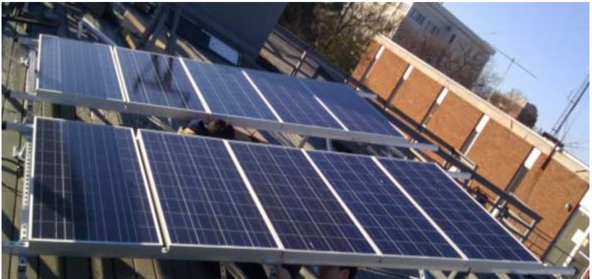
Figure 5.2: Photograph of grid-connected PV system.
