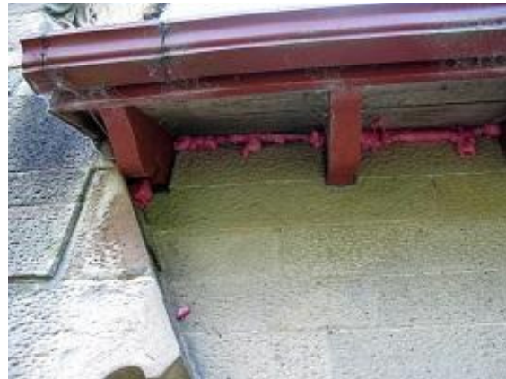
Damaged bat roost © John Haddow
