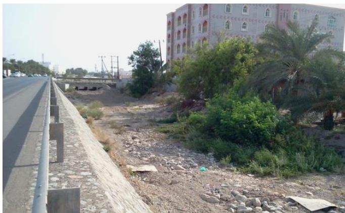
Figure 8.9: The bridge depicted serves one building and caused flooding in 2007 Source: Author's own
