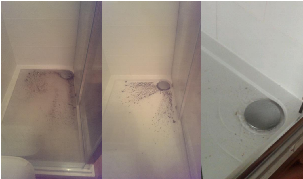
Figure 2. 13, Effect (in ground floor flat shower room) of positive pressure transient generated upon the discharge from the top floor bath in a two pipe system.
