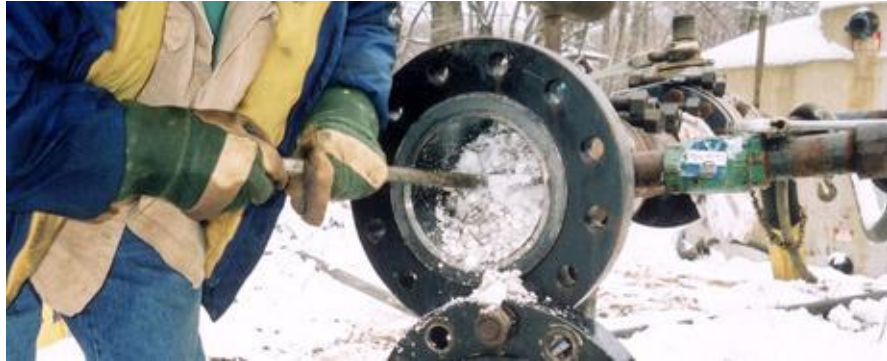
Figure 1.17: Gas hydrates removed from a pipeline [1.41]
