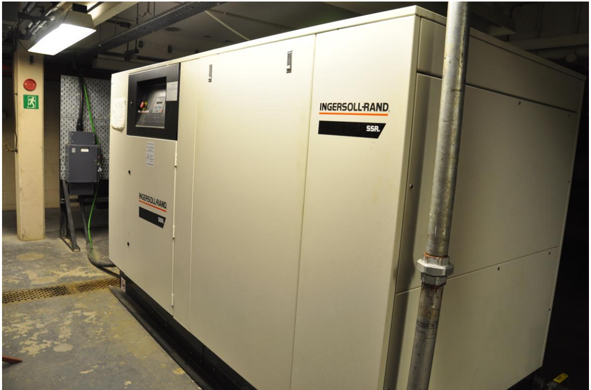
Figure 3.18: The Ingersoll-rand SSR M110 compressor supply compressed air to test section
