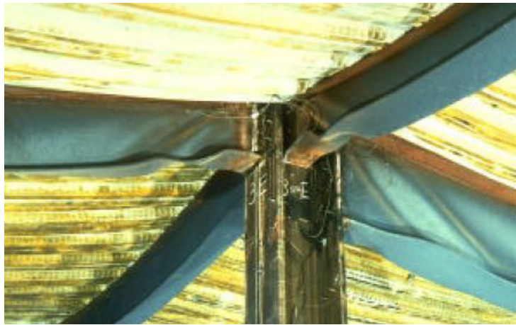
Figure 1.1 Failure of plate-girder beams initiated by shear buckling of the webs (Newman et al, 2001)
