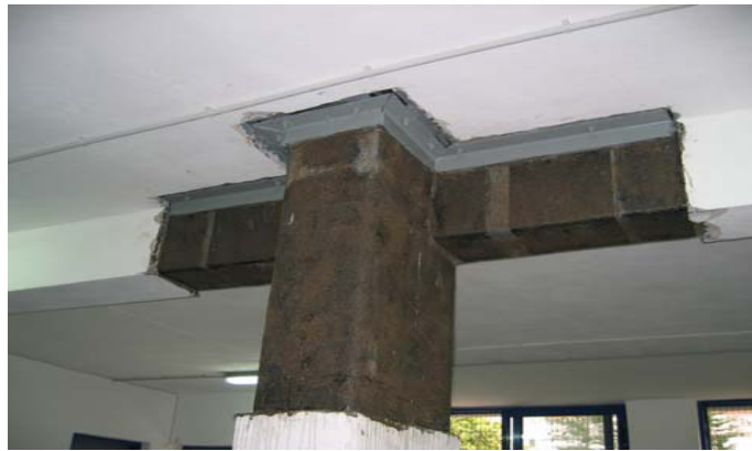
Figure 2.15 CFRP-confinement of column-beam joints at Aigaleo football stadium in Athens, Greece (Motavalli & Czaderski, 2007)
