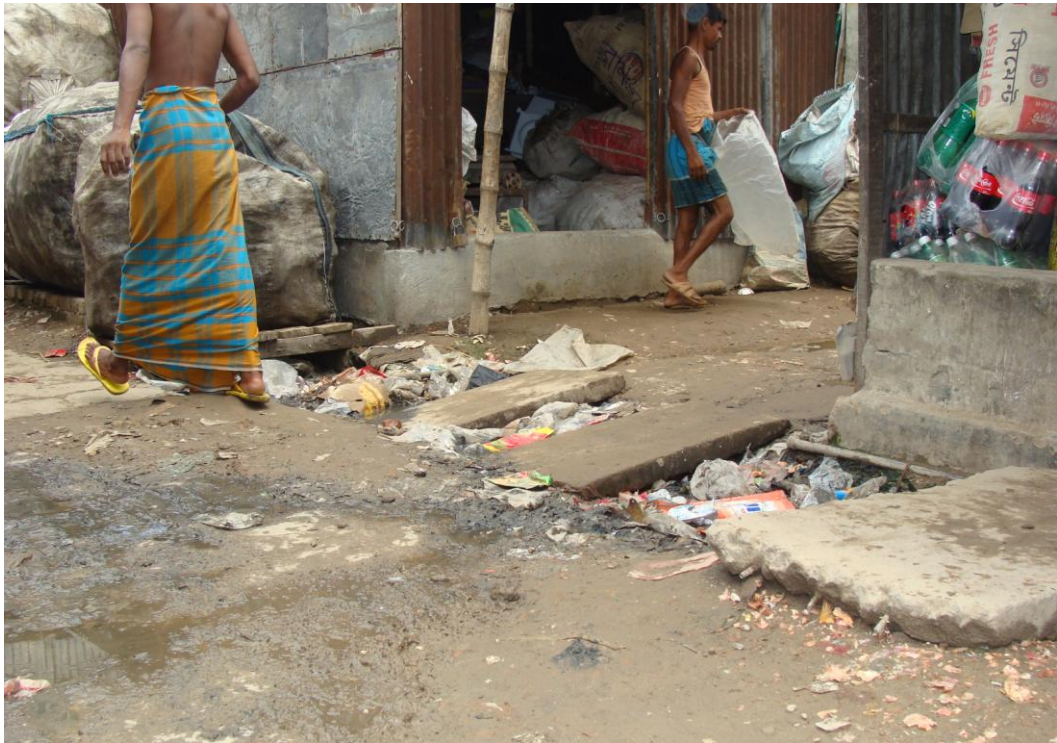
Figure 5.11: Poor Maintenance of Existing Drainage System in Karail slum
