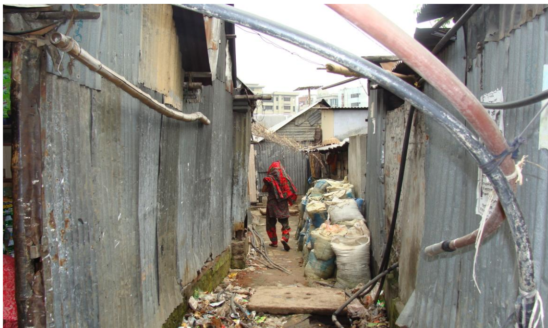
Figure 5.17: Water Supply Pipeline Network in Karail Squatter Settlement
