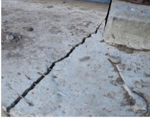
Cracks in tram track bed
