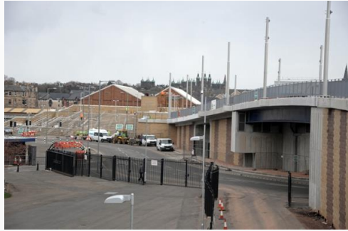
Completed Tram Bridge over Roseburn Street leading to Murray field tram stop
